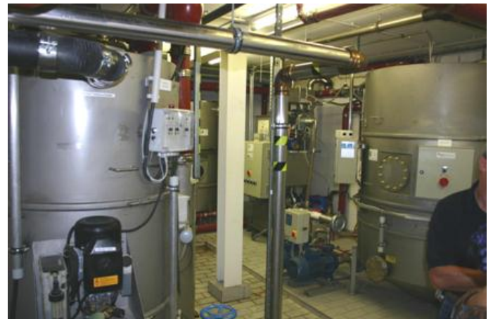
Fig. 5: Greywater treatment facility in KfW Ostarkade (Photo: GTZ)
