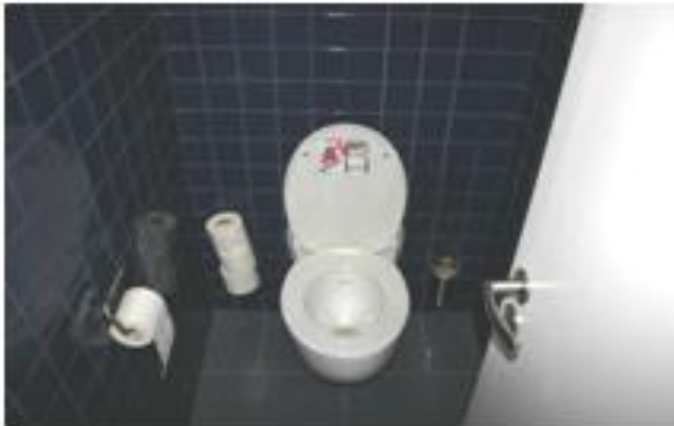
Fig. 2: Vacuum toilet in KfW building ostarkade (photo: gtz)
