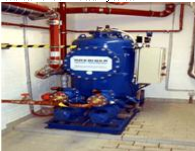
Fig. 3: Vacuum pumping unit (Photo: KfW)
