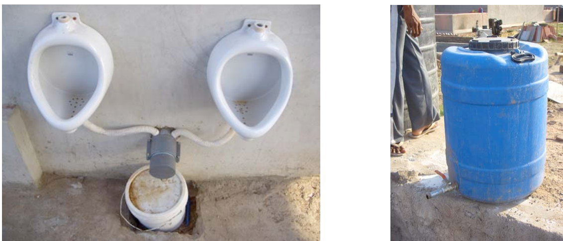
figure 17: Urinals for males and transportable collection tank (left) and storage/hygienisation tank (right)
