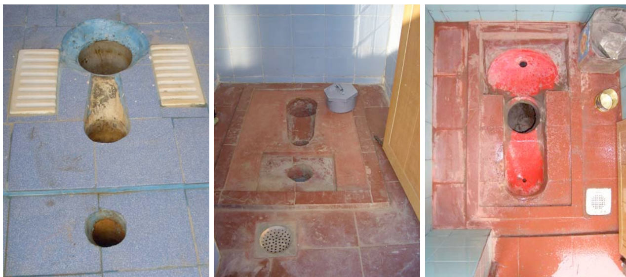
figure 16: “3-hole system” at ACTS eco-friendly demonstration toilet in Rajendra Nagar, Bangalore (left), “3-hole system” at Navsarjan Primary School in Dhandhuka taluka (center) and prefabricated squatting pan that allows source-separate collection of urine, feces and anal cleansing water (design supported by UNICEF) (right)
