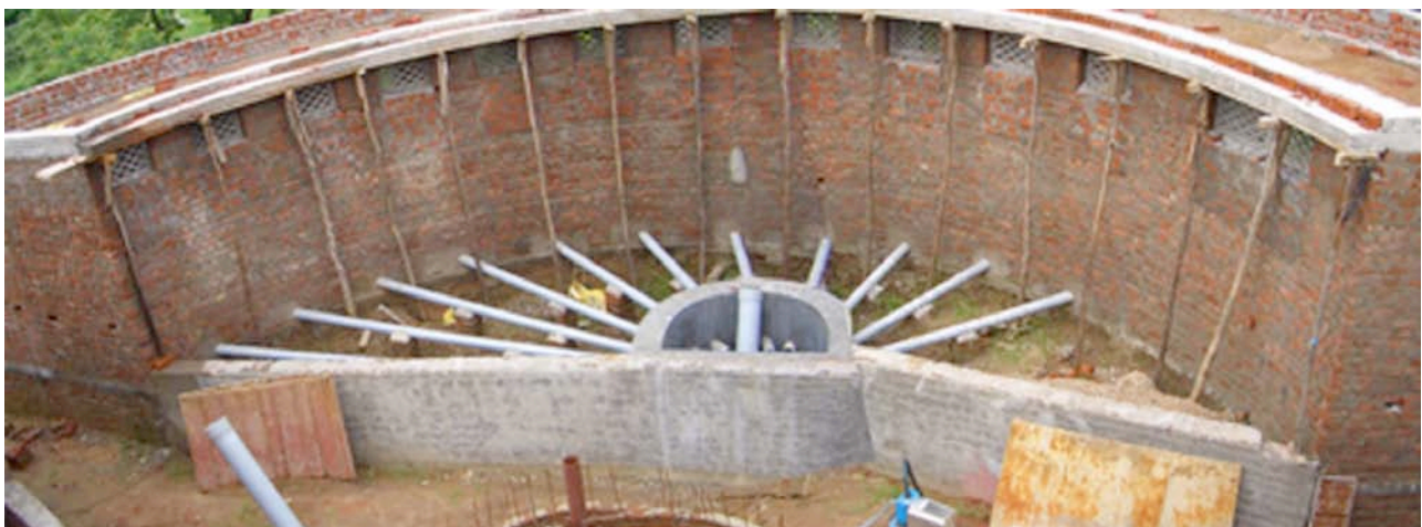
figure 9: Night-soil based biogas plant [clockwise from top left: conceptual sketch of toilet linked biogas system; view of new toilet block; top view of hoppers and biogas plant (under construction); rear view of toilet cabins depicting individual blackwater disposal pipes (before refilling with soil and landscape gardening); picture of “pour-flush” squatting pan with water seal (“P”-trap)]
