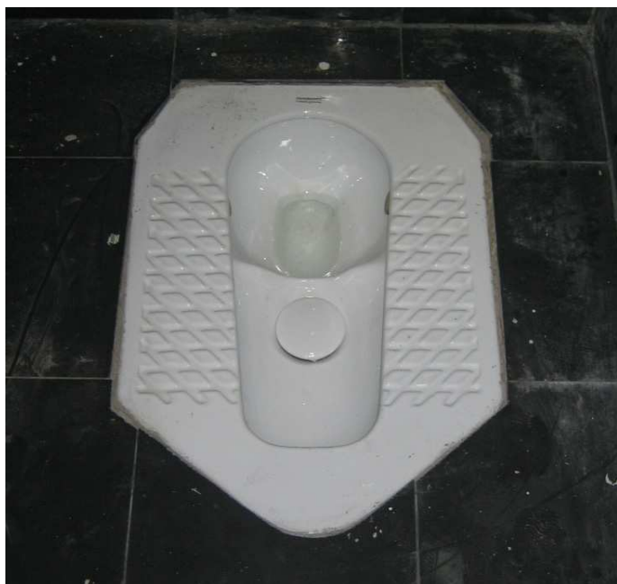
Fig. 4: Urine-diversion vacuum squatting toilet in the Sino-Italian Environment & Energy Building (source: EnviroSystems)
