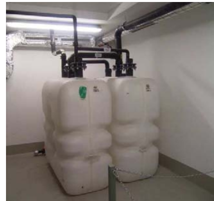
Fig. 7: The two plastic urine tanks (currently bypassed) in the school building's basement have a capacity of 1.5 m 3 each (source: OtterWasser GmbH).
