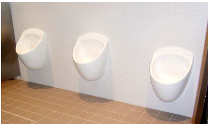
Fig. 6: Waterless urinals for boys from the Austrian company Hellbrok in the school building – hung lower than for adults (source: OtterWasser GmbH).
