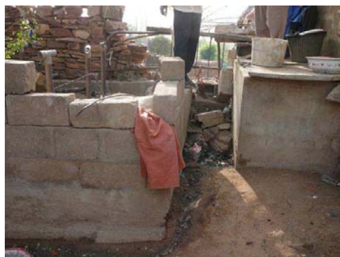
Fig. 4: The same location as Fig. 3: greywater garden on the left side with leaking water from broken pipe (source: Stefan Hofstetter, March 2009).
