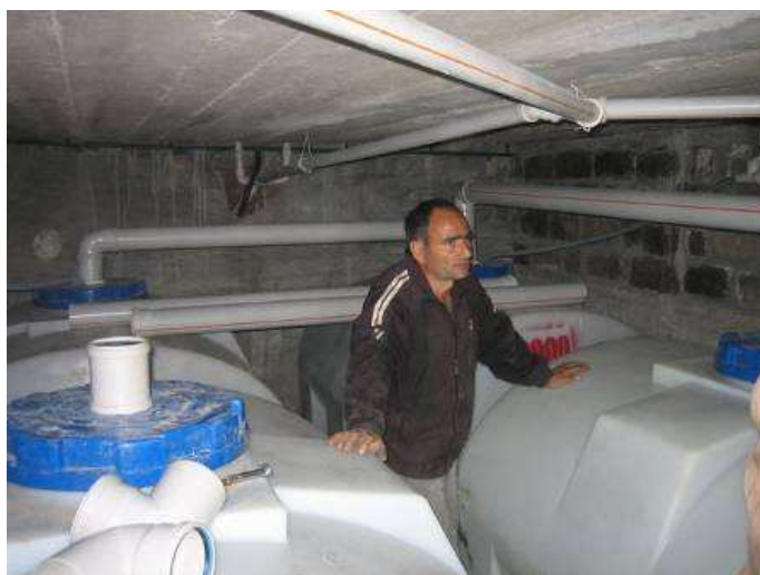
Fig. 11: Urine tanks (4 x 2 m 3 ) in the basement of the school (source: AWHHE, 2006)
