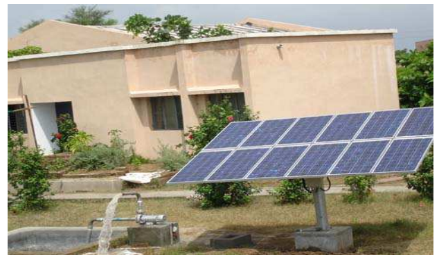
Fig. 8: Solar panel and water pump (source seecon GmbH, which year?)
