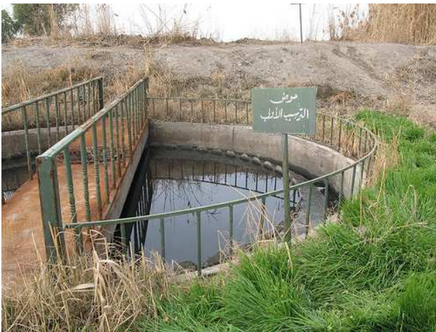
Fig. 7: Circular primary settling tank at Haran Al-Awamied treatment plant. Source: E. v. Münch, Jan. 2009.
