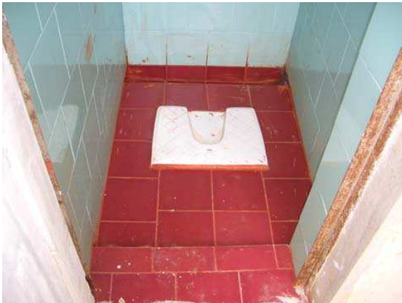
Fig. 6: View of ladies squatting urinals, which are now water flushed (source: seecon GmbH, which year?)
