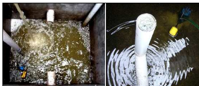
Fig. 4: Outlet of the blackwater compost filter (pre-treatment) (left) and effluent of the constructed wetland (papyrus reed bed) for blackwater treatment (right).
