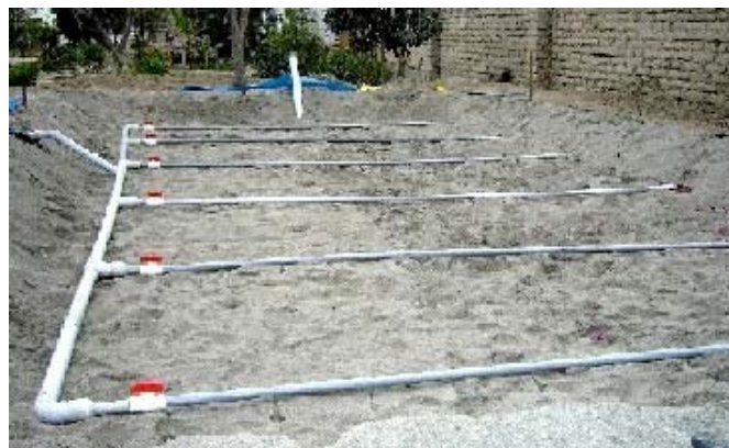
Fig. 18: Distribution system on the second constructed wetland (for blackwater treatment) before planting, showing valves on the left (in red) to avoid clogging (intermittent loading).
