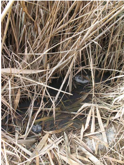
Fig. 9: Overloaded, water-logged reed bed towards outlet section of reed bed (source: E. v. Münch, Jan. 2009)
