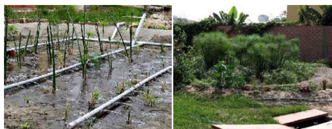
Fig. 5: Vertical flow constructed wetland for greywater treatment during pumping (a day after planting and before the protection of the distribution pipes with a 10 cm gravel layer) (left) and after two months, with storage tank for irrigation of treated greywater (right).
