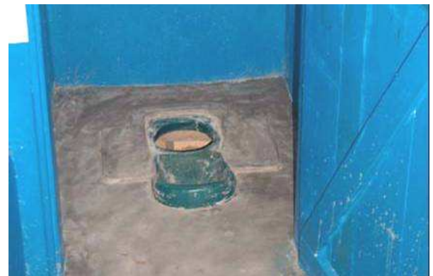
Fig. 5: Interior of a students' UDD toilet showing UD squatting pan (source: EcoSan Club, year?)
