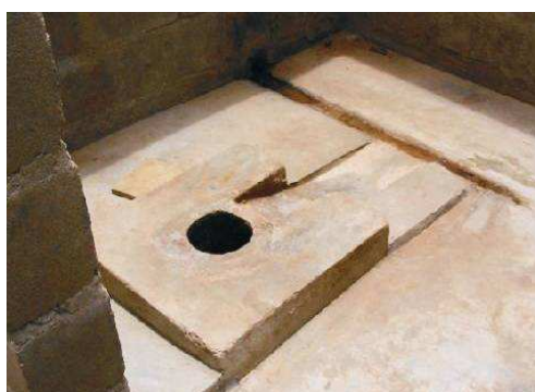
Fig. 6: Latrine urine-diversion squatting pan, where urine drains away to the drainage at the right (source: GTZ, 2002).
