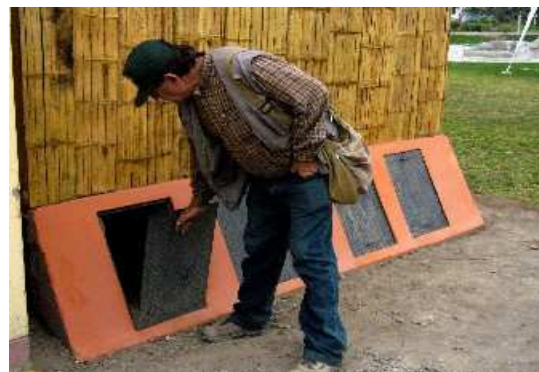
Fig. 11: Two double-vaults for faeces collection at the backside of the UDDT building (4 vaults in total).
