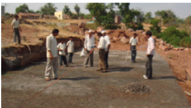
Fig 5: Horizontal Flow Constructed Wetland for...? (under construction) Where..? Month, year? (photo: N. Zimmermann)
