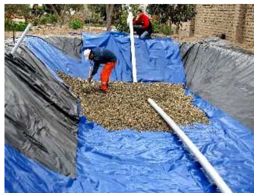
Fig. 3: Drain tube on the base of the constructed wetland for blackwater treatment during covering with gravel. To avoid perforation caused by the gravel, the 0.5 mm PVC liner (in black) needed a special protection. A second liner (in blue) was put inside. 1
