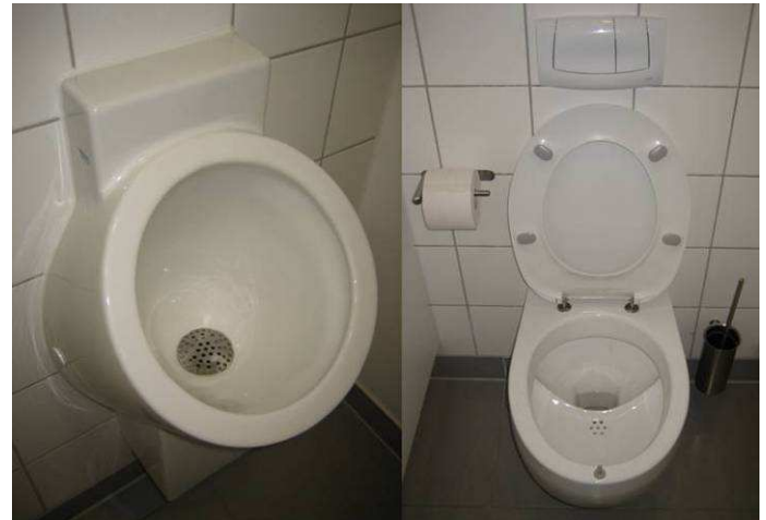
Fig. 4: Left: waterless urinal (Keramag). Right: urine-diversion flush toilet (Roediger) at GTZ main building; note the two buttons for flushing: the small one is for the urine flush, the larger one for the faeces flush (source: L. Ulrich, January 2009).
