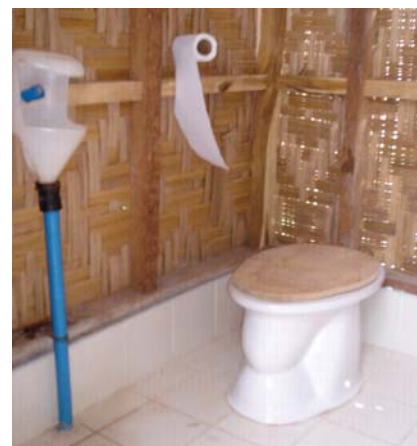
Fig. 3 Ecosan UDD toilet (painted concrete pedestal) at Libertad Municipality (photo: E. Sayre, March 2008)
