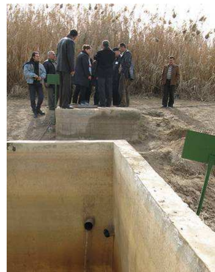
Fig. 12: Foreground: effluent tank with two effluent pipes discharging from the two reed beds. Background: reed beds and group of trainees (source: E v. Münch, Jan. 2009).
