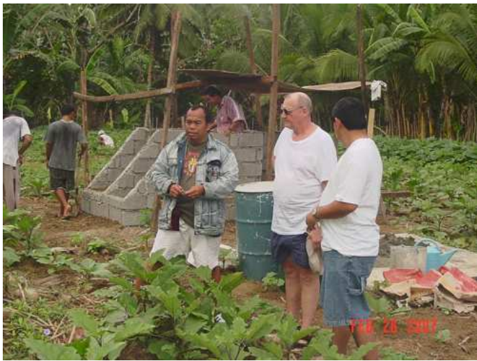
Fig. 7 Elmer Sayre with 2 visitors inspecting construction of a UDD toilet and a garden for product reuse at Libertad Municipality (photo: WAND, Feb 2007)
