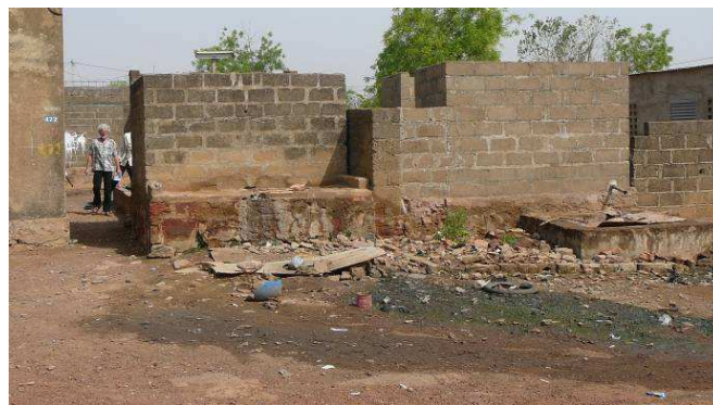
Fig. 8: Former desiccation (drying) chambers of UDDTs have been converted into pits to collect faeces and to be pumped empty when full (source: Stefan Hofstetter, March 2009).
