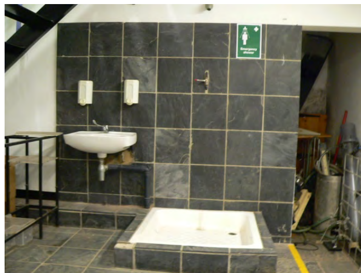
Emergency Wash Station and Shower
