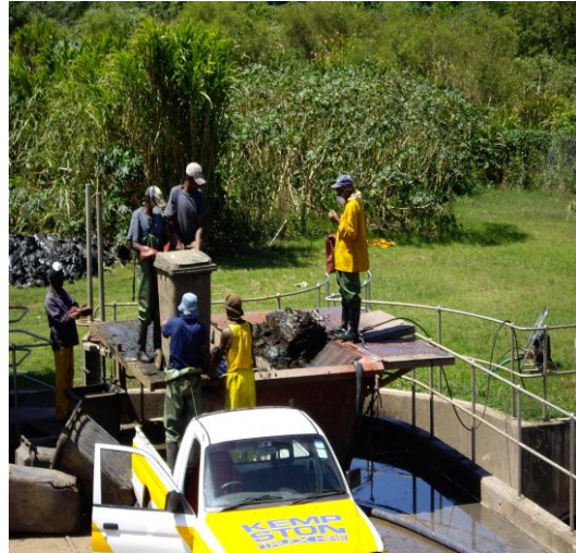
(b) screening of sludge content at treatment works.
