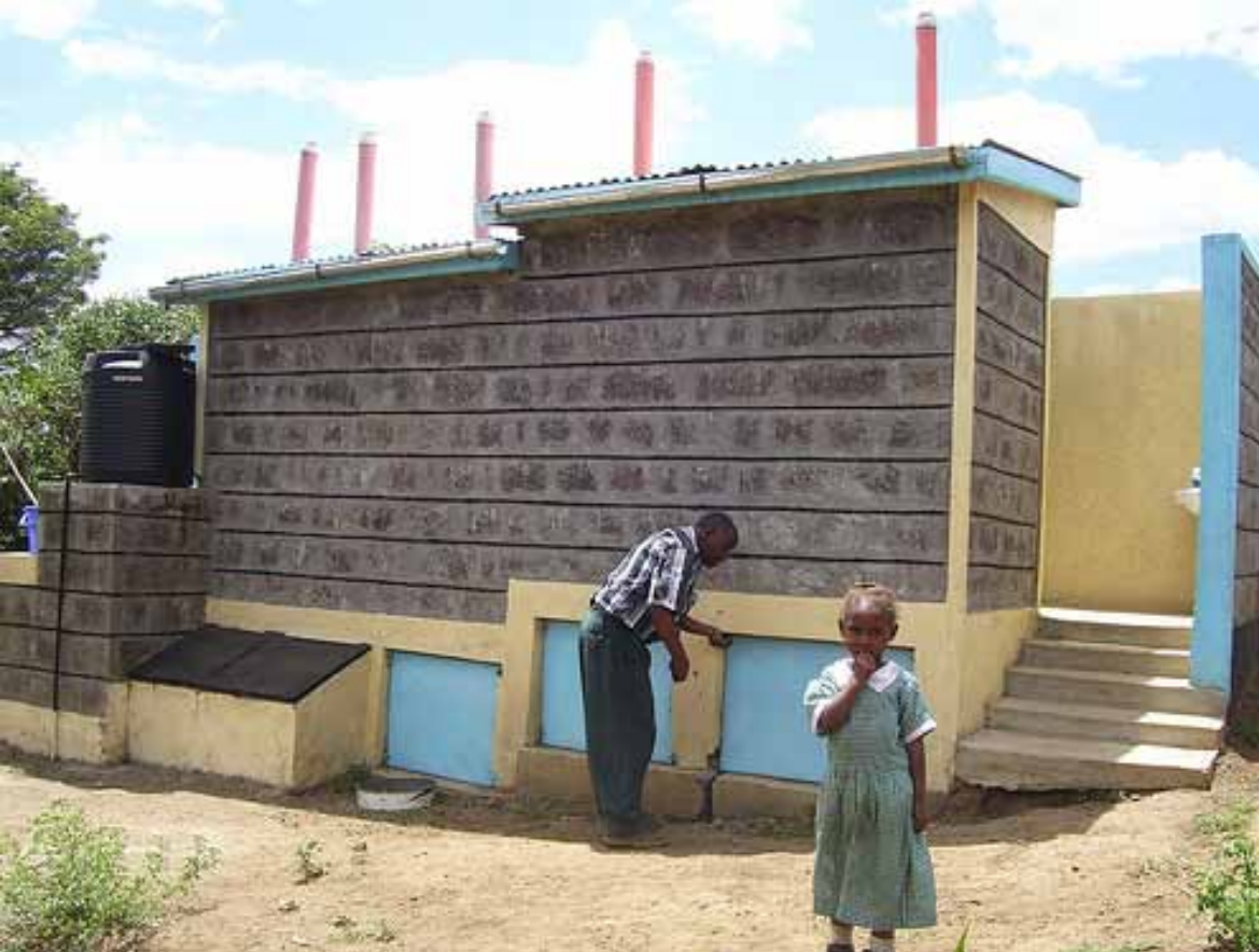
Back of UDD toilet block at nursery school in Nakuru, Kenya (ROSA project)
