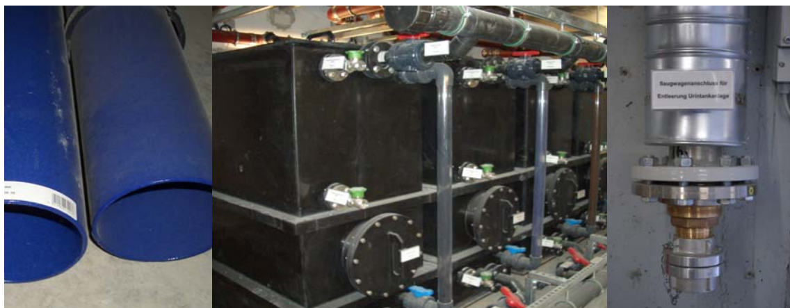
Figure 5 Pipes of cast iron with enamel coating (left), urine tanks (middle), and docking station for tank trucks (right) (source: GTZ)
