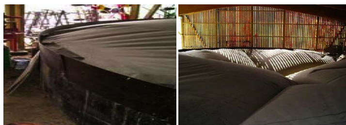
Figure 4: Digester Tanks (Photo: Wang)
