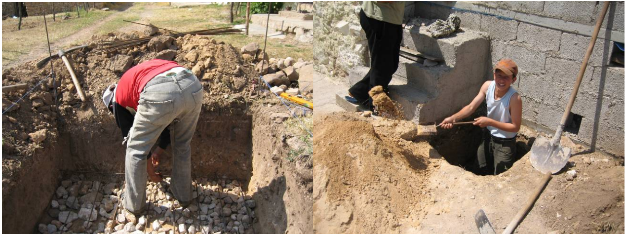
Fig. 62 : Iron for floor of wetland (left) and excavation for urine tank (right) at Jane
