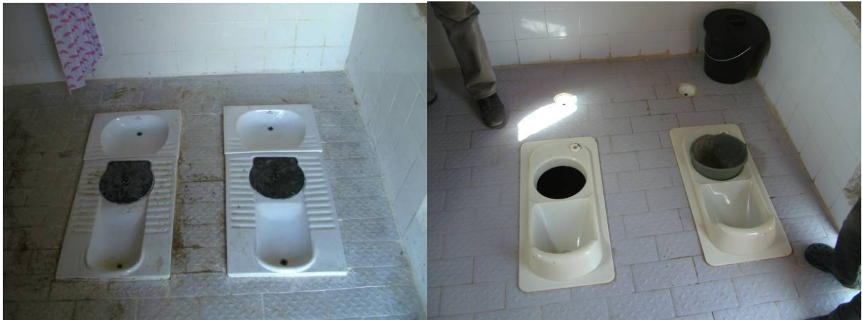
Fig. 2: examples of urine-diversion slabs with anal cleaning 1
