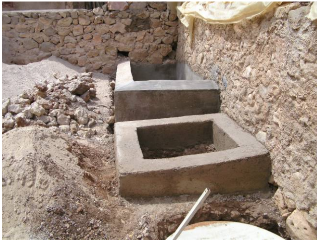
Fig. 90 : Walls for Urine-tank (front) and wetland for Greywater (background) at Khaled
