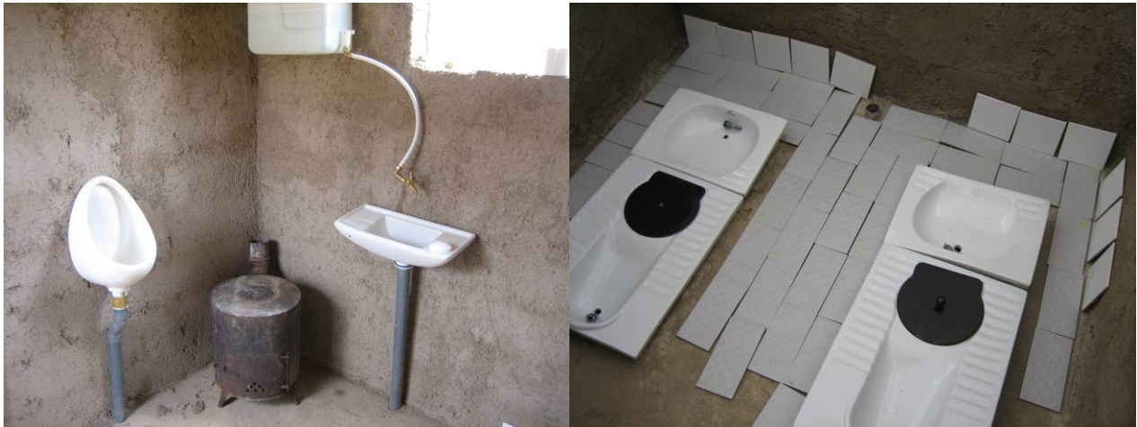
Fig. 61 : Provisional sanitary installations at Ferhaoui (left) and Ahnuch (right)
