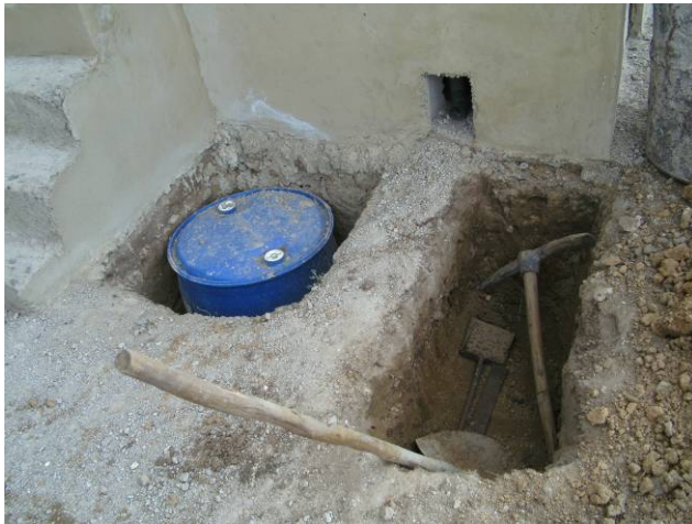
Fig. 79 : Urinetank (left) and beige-water-infiltration (right) at Jane
