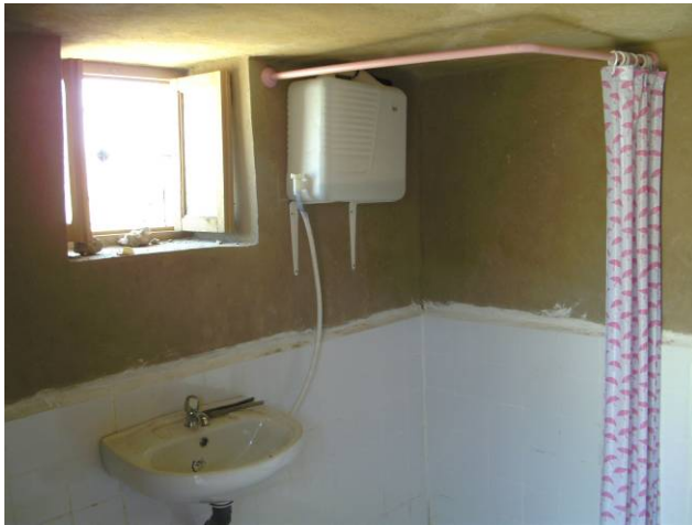
Fig. 105 : Water-tank, sink and place for shower at Khaled
