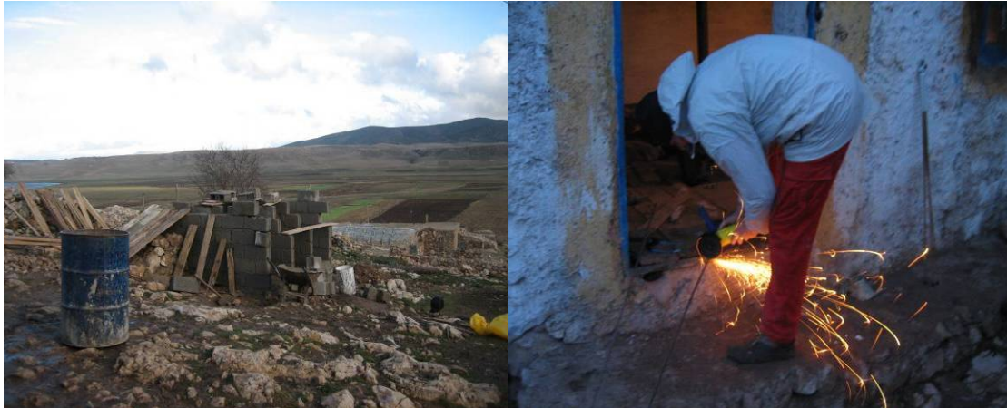
Fig. 28 : Preparing lower formwork and cutting iron for armour of the ground plate
