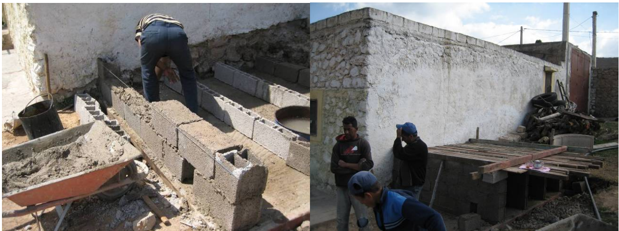
Fig. 40 : Faeces-chamber-walls at Jane, note space for pipes (left); formwork for plate (right)
