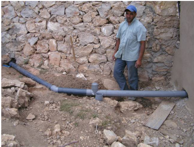
Fig. 103 : Greywater-pipe from kitchen to wetland at Ahnuch
