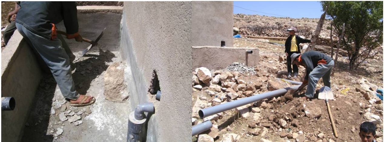
Fig. 83 : Repair of broken sealing of wetland (left) and digging for urine-pipe (right) at Ferhaoui
