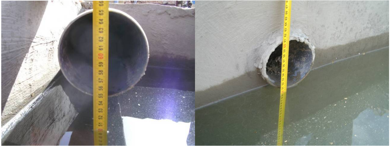
Fig. 93 : Influent-pipe exactly 5cm higher than effluent-pipe at Jane
