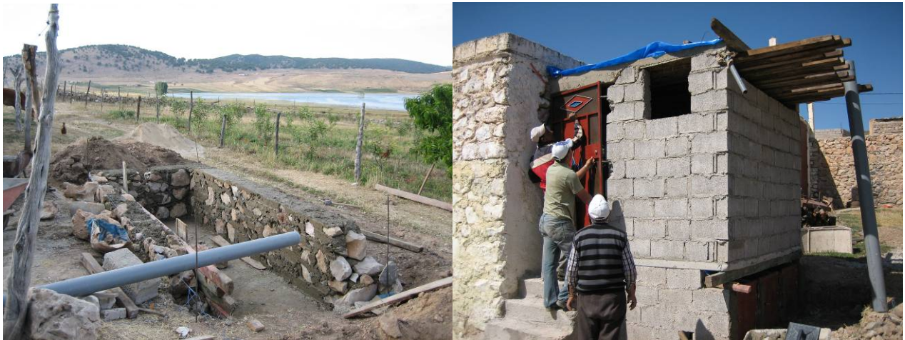
Fig. 67 : Building walls of wetland (left) and installation of doors (right) at Jane
