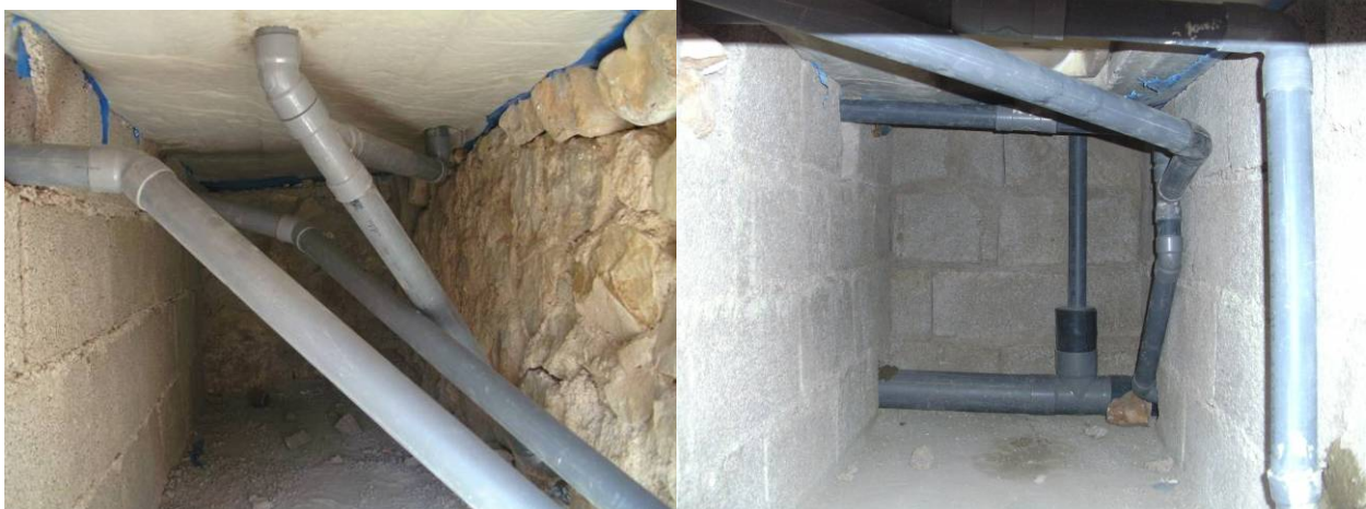
Fig. 104 : Pipes at Khaled below shower (left) and in faeces-chamber at Ahnouch right
