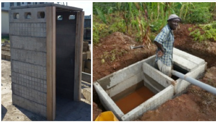
Figure 2. Pre-fabricated superstructure with low volume flushing toilet. The toilet superstructure is constructed from interlocking cement blocks enabling faster construction (left). The pour flush prototype uses low volumes of flushing water which goes into sumps (right). The same building blocks can be used to build the sumps. Photos by Water for People Uganda.
