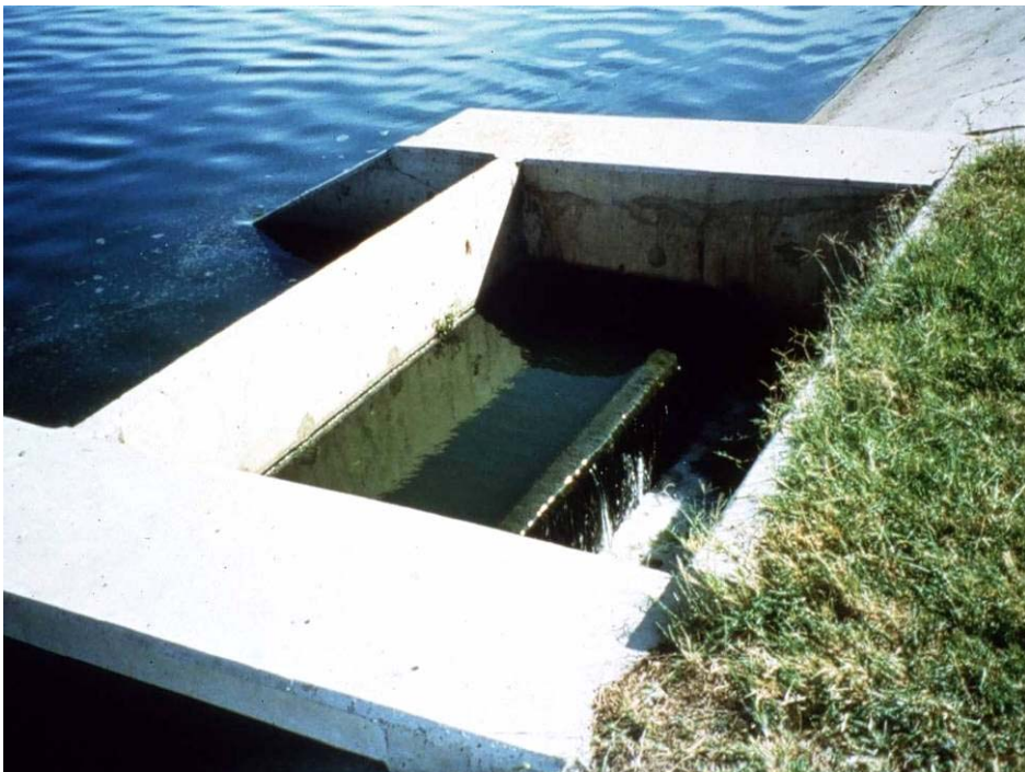
Figure 9. Pond outlet weir with integral scum guard.
