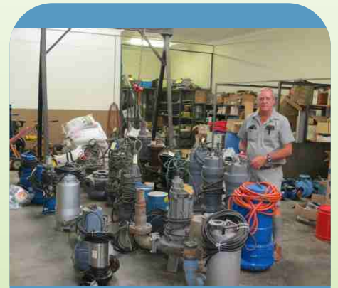
Ben du Plessis with spare pumps in the workshop
