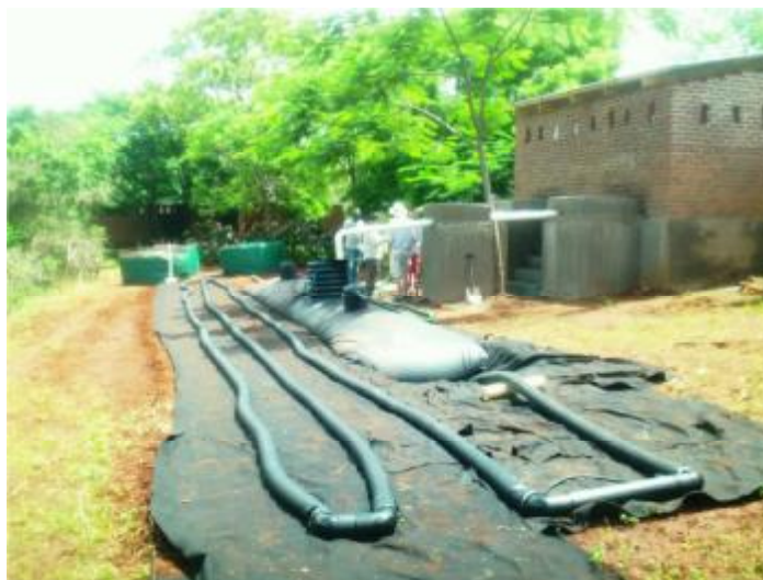
Sludge Treatment: Flexigester Trials - Malawi. February 2013
