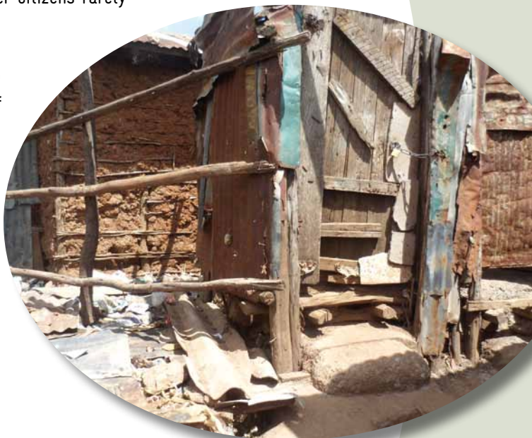
Inaccessible pit latrines in Mathare
