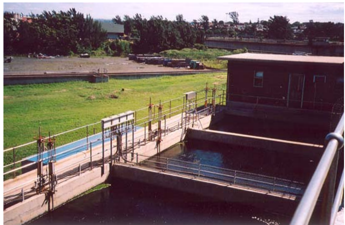
Abbildung 23: Veolia Wastewater Treatment Plant in Durban
