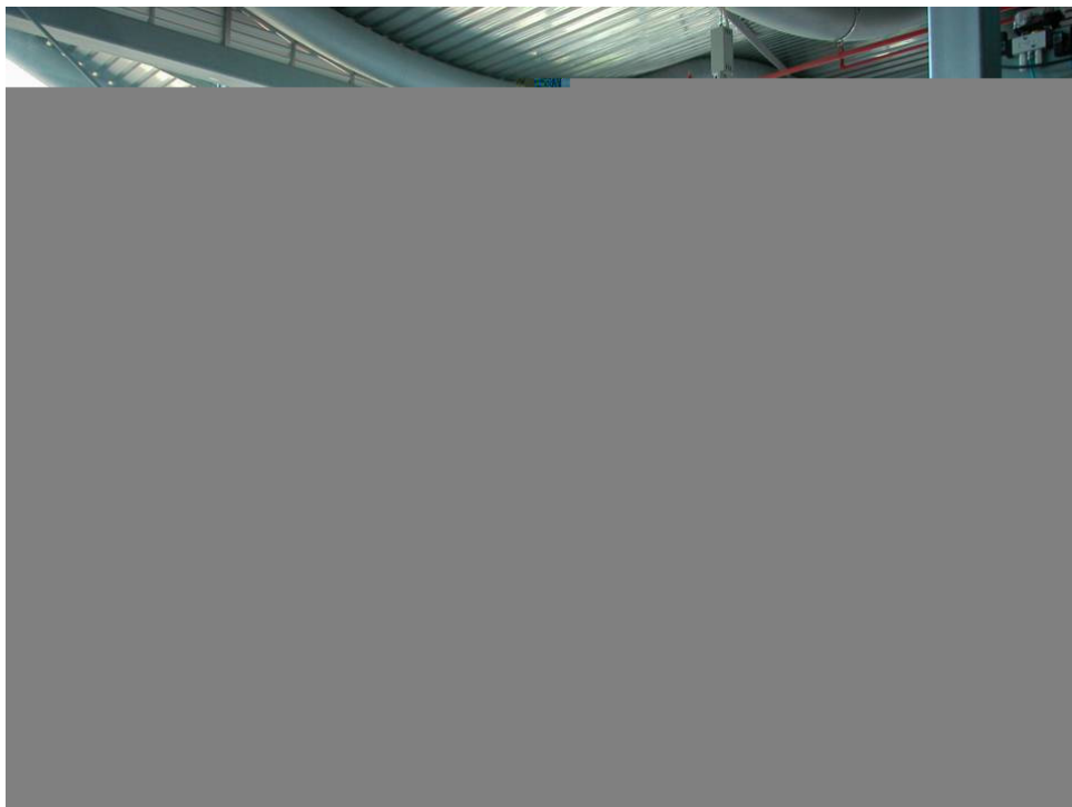
Figure 9.11: Reverse Osmosis Units at the NeWater water recycling scheme in Singapore
