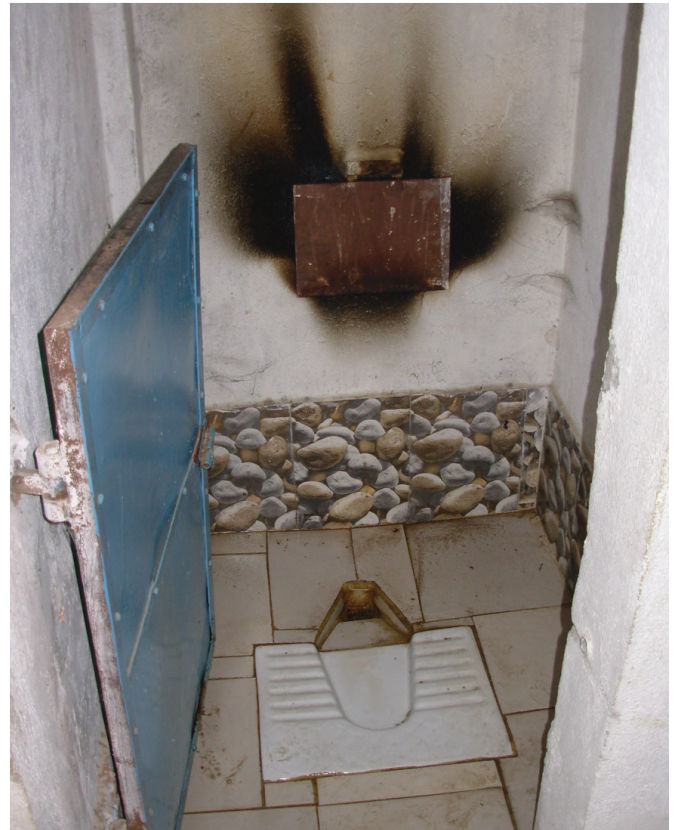
Waterless urinal with sanitary padding incinerator
