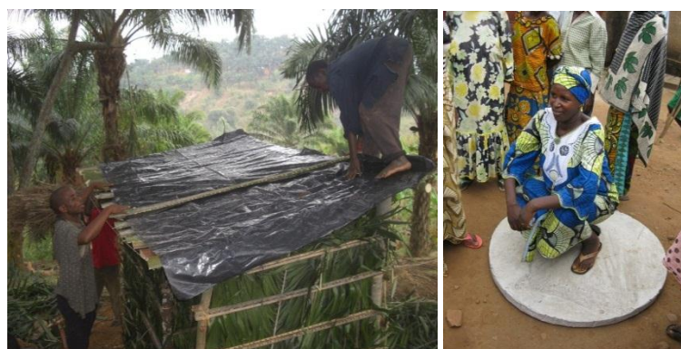
Figure 2. Left. Construction of simple composting latrines called AKASUGA in Burundian language.; Right. Testing of dome slabs during awareness campaigns. Photos by F. Reman/GIZ-ProSecEau (2013)
