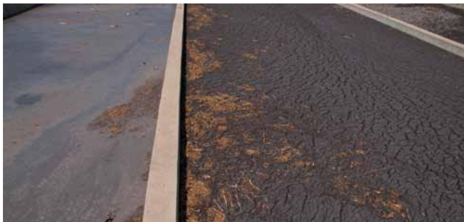
Figure 7.2 Freshly loaded and partially dewatered faecal sludge on unplanted drying beds at Niayes faecal sludge treatment plant, Dakar, Senegal (photo: Linda Strande).
