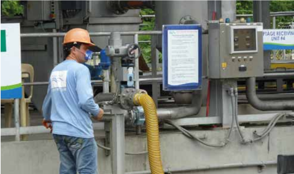
Figure 4.16 Automated faecal sludge receiving station at Manila Water's South Septage Treatment plant, Manila, Philippines (photo: WSUP, Sam Parker).
