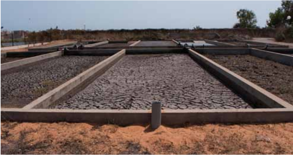
Figure 3.4 Drying beds at Niayes faecal sludge treatment plant, Dakar, Senegal (photo: Linda Strande).
