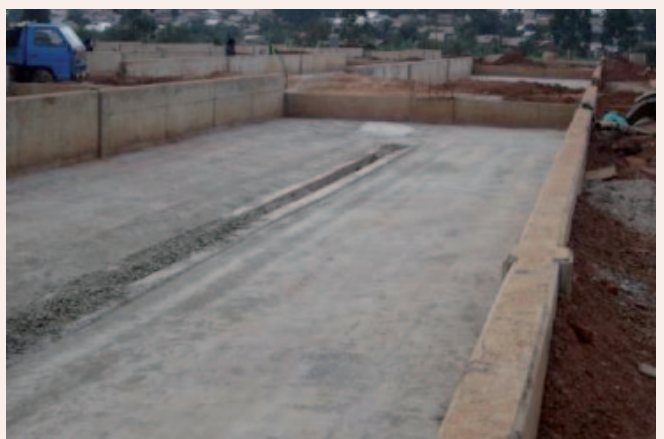
Figure 3: Drying beds in construction at the new faecal sludge treatment plant in Kampala.
