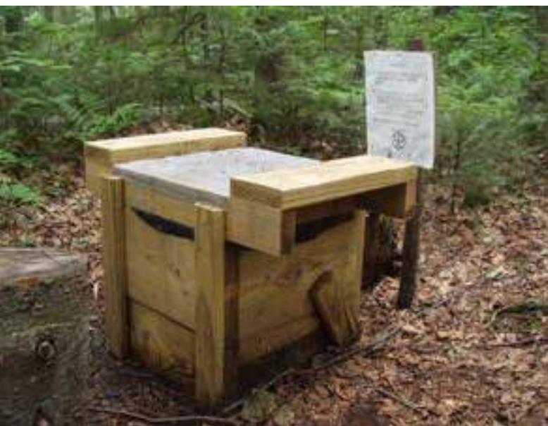
Gray Water Trickle Filter - note side tables for holding dishes
