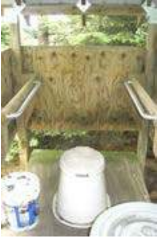
This accessible privy is missing the T-Turn around clear space
