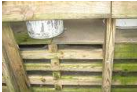
Moldering Crib - note plastic riser placement
