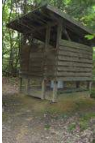
This accessible privy is missing a transfer platform
