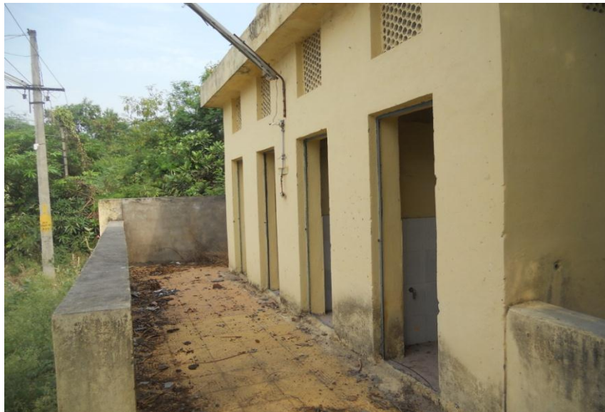
Dysfunctional community toilets
