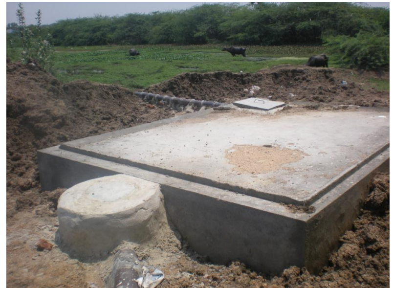
Badly designed septic tanks
