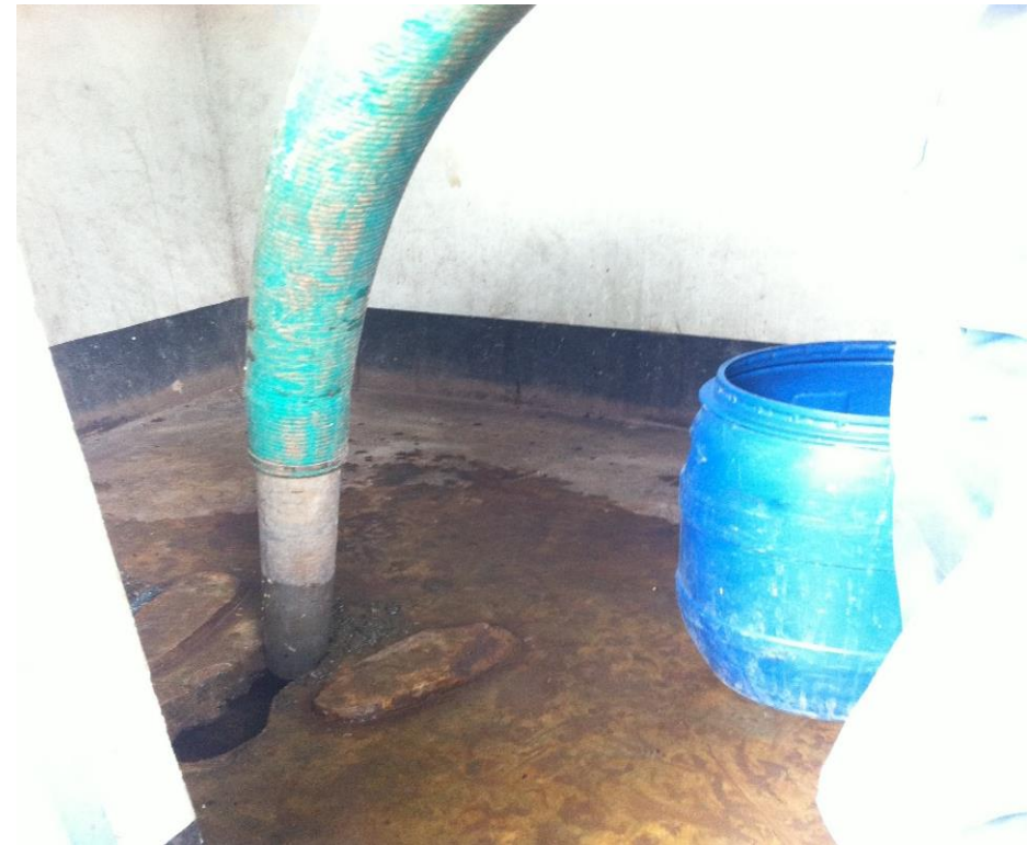
Desludging after excessive hydration due to presence of hard sludge
