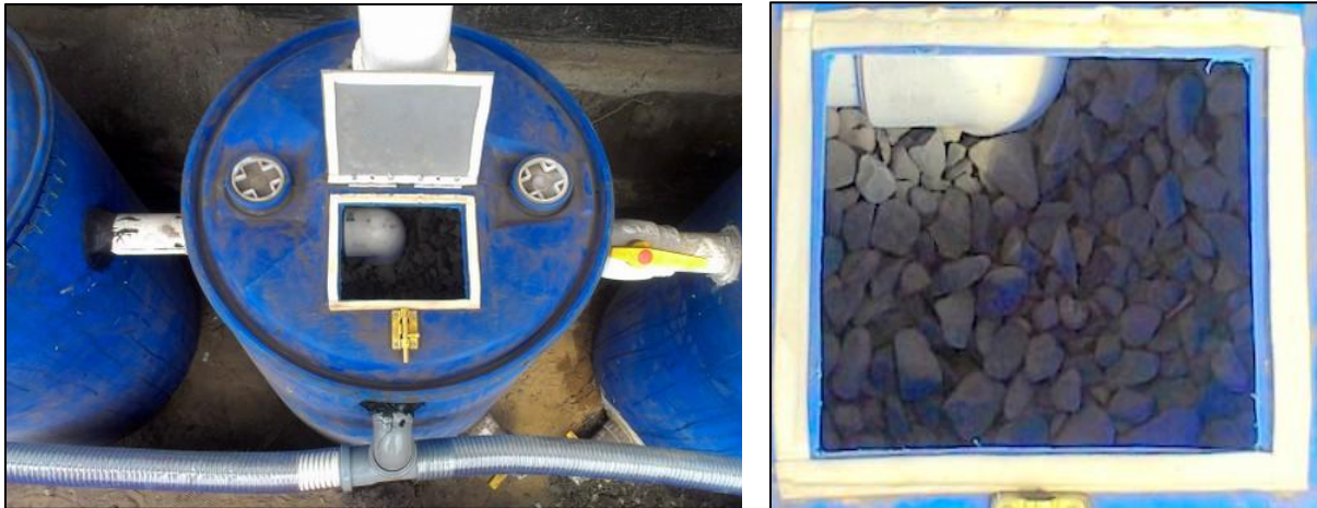
Figure 17: One compartment out of three of the upflow roughing filter (UFRF) at the GHTU (left) and filter media inside during construction (right) (ACF, 2013).
