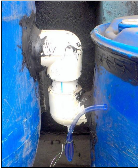
Figure 32: Connecting pipe between barrels supplied with a flexible hose for sampling (ACF, 2013).
