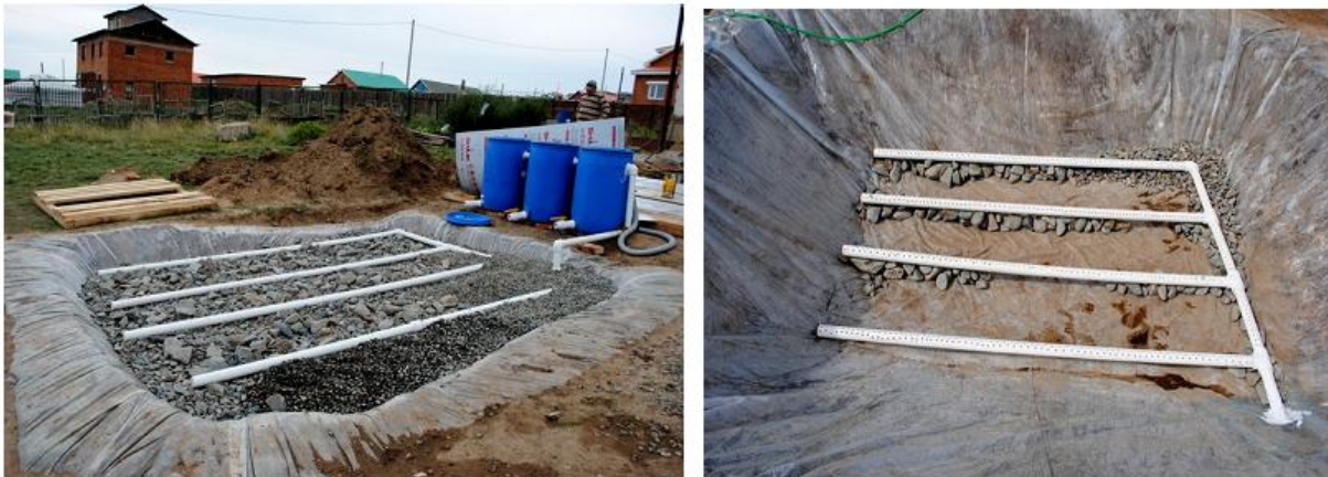
Figure 22: Distribution system with septic tanks (left) and drainage system (right) during construction of the CW at the IBU (ACF, 2013).
