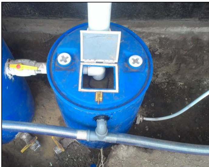
Figure 24: The slow sand filter at the GHTU (ACF, 2013).
