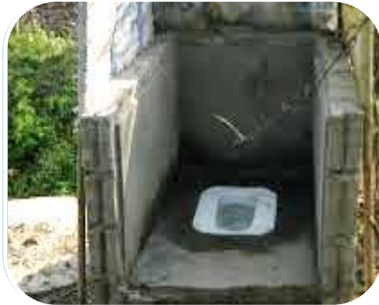
Unsafe containment of sludge at source
