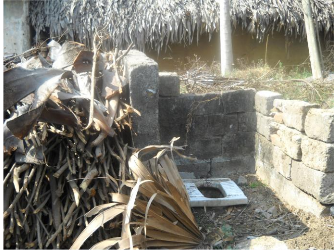
TSC toilet in un-usable condition (Odisha)
