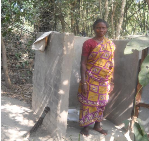
TSC toilet with low walls and no roof. Repondent wants to upgrade to higher walls and a roof (Odisha)
