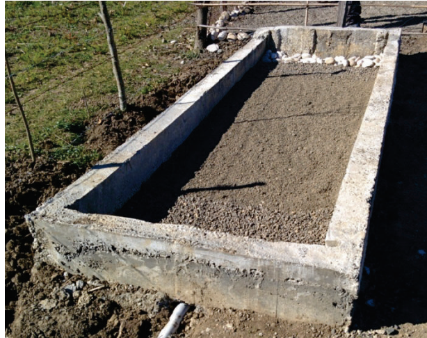
Figure 7: A horizontal greywater filter in the project region, between construction and planting.
