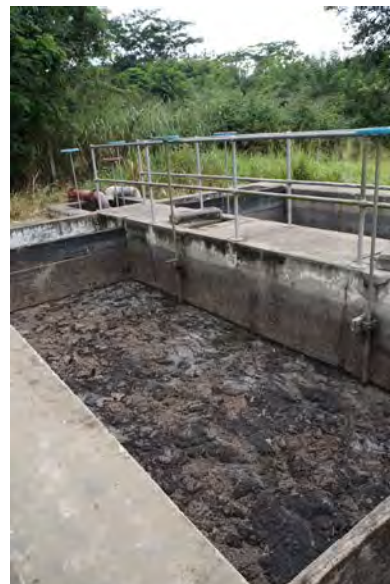
Sludge drying bed at KNUST Sewage Treatment Photo credit: Claire Furlong
