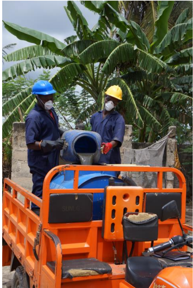
FS transfer to storage tank for transport. Photo credit: Moritz Gold
