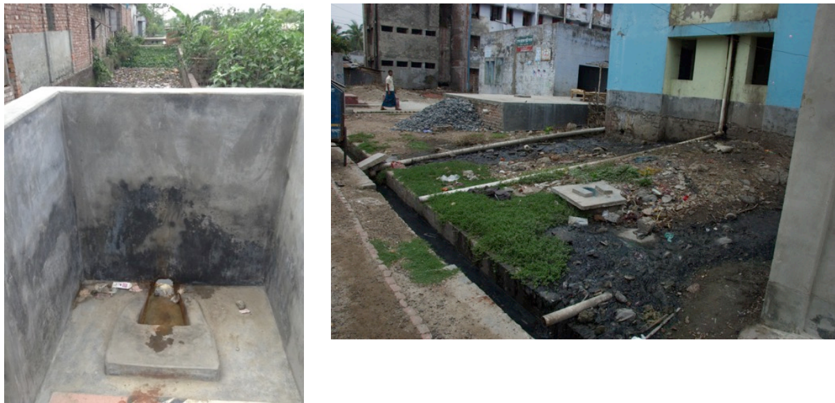
Figure 10: Public toilet connected to open ground (left) and community building blocks connected to open drain (right). Photos: Arief Gunawan (left), Lars Schoebitz (right).
