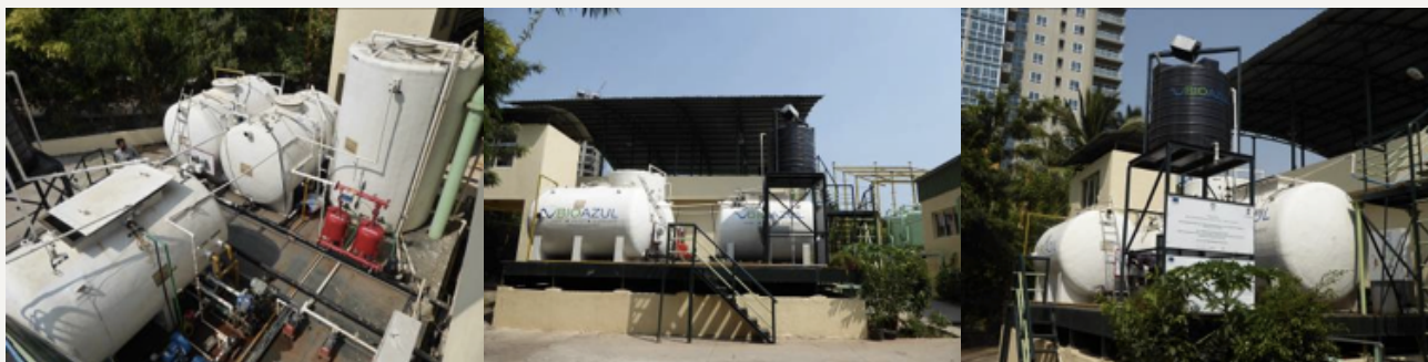
Figures 5, 6 and 7: Combined wastewater treatment system (SBR and MBR) for wastewater reuse in Amanora Park Town (source: BIOAZUL, 2015)
