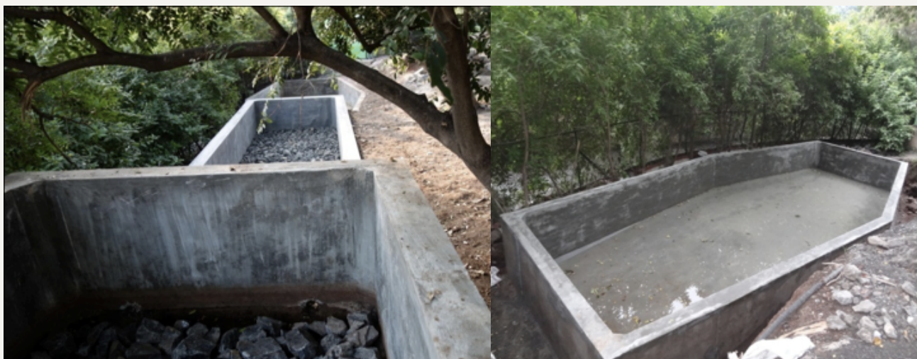
Figure 5 - Overview of treatment system (left) and treated water pond (right) under construction.
