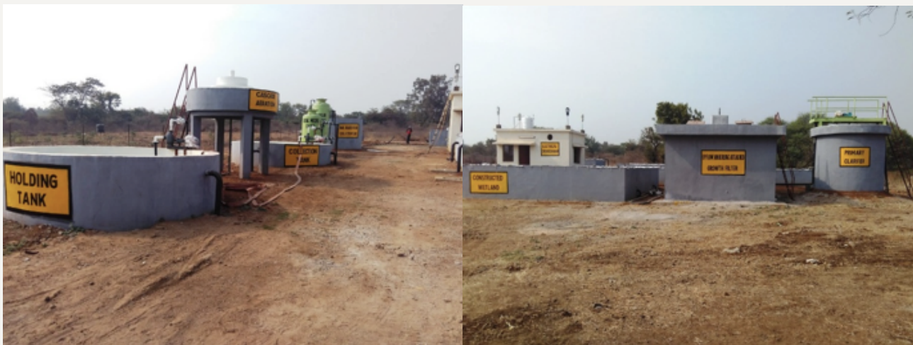
Figure 4: Overall view of main treatment line at OFAJ, Nagpur after completion of the implementation
