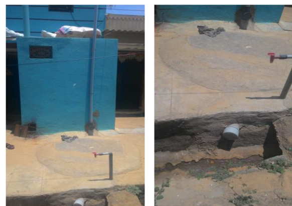
Figure 1: Toilet connected to pit with opening for emptying septage (Source: Rahul/CSE, 2015)
