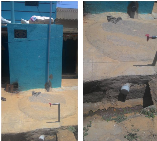
Figure 2: Toilet connected to a pit with opening for emptying septage (Source: Rahul/CSE,2015)
