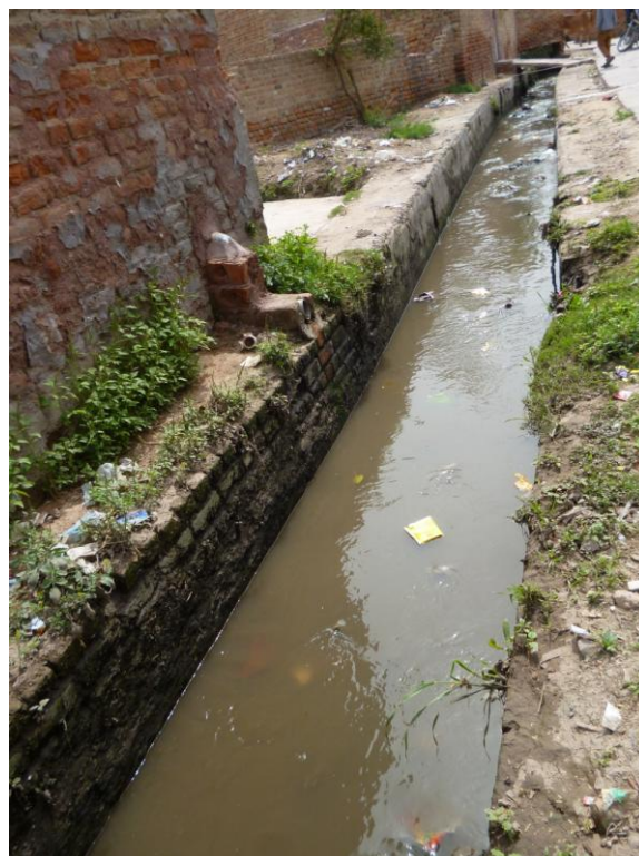
Figure 1: WC to open drains (Source: Shantanu & Rahul/CSE, 2015)
