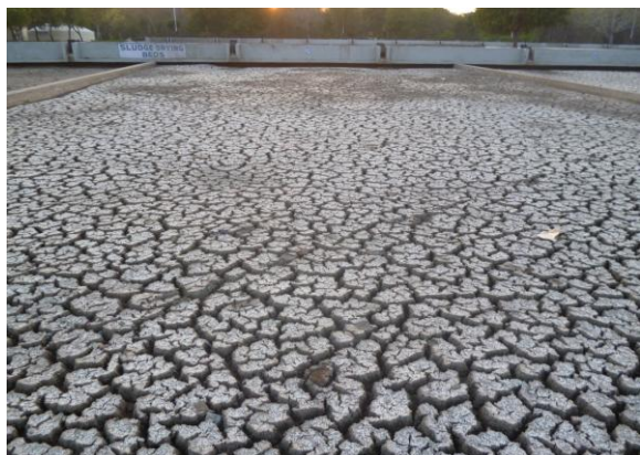
Figure 2: Sludge drying bed - UASB technology 78 MLD STP in Dhandupura (Source: Rahul/CSE, 2015)
