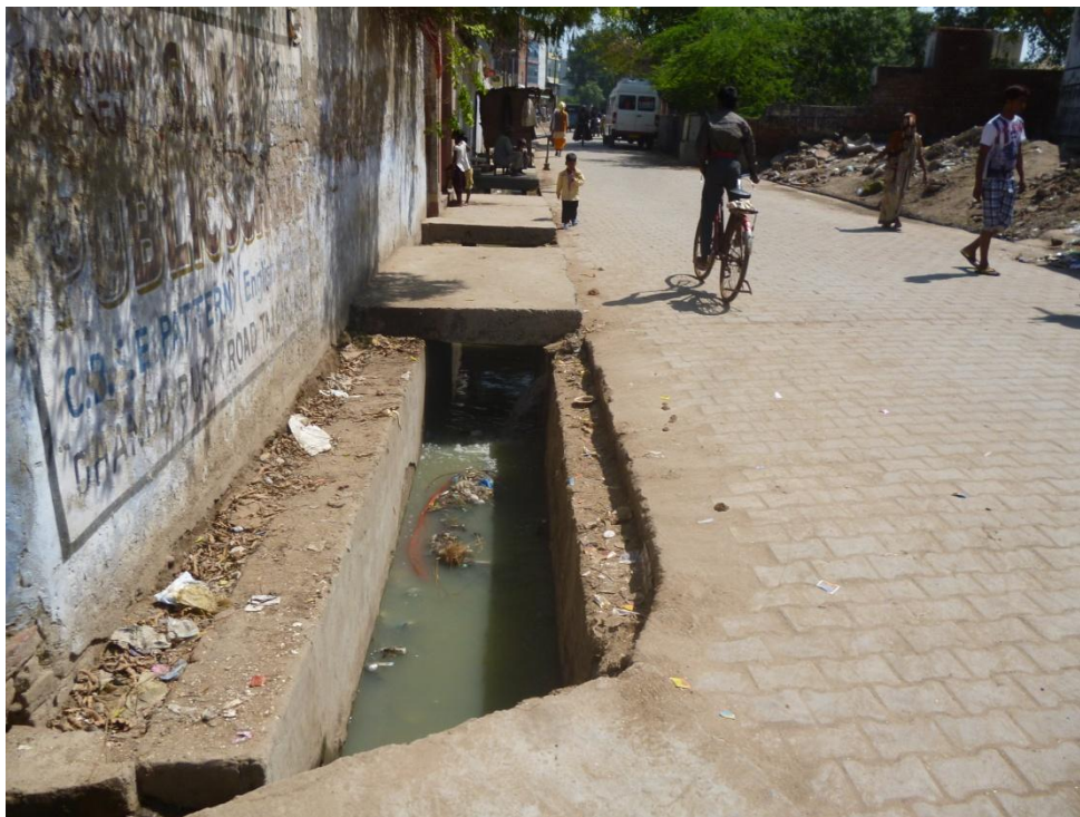
Figure 8: Open drain in the city (Source: Shantanu/CSE, 2015)
