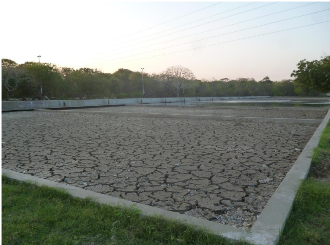
Figure 6: Sludge drying bed in Dhandupura STP (Source: Rahul/CSE, 2015)
