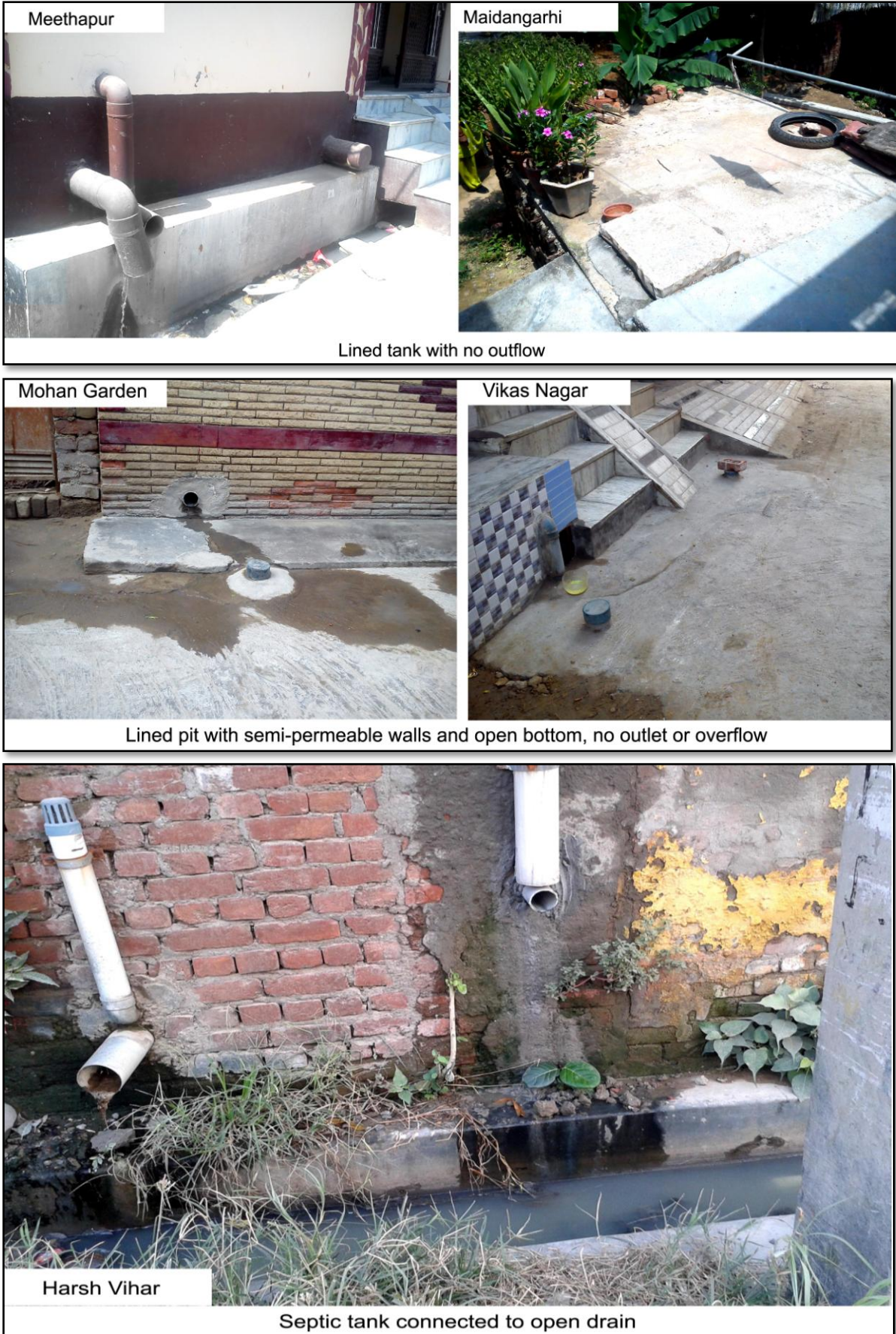
Figure 3: Type of containment systems observed during field based study (Source: Anil/CSE,2015)
