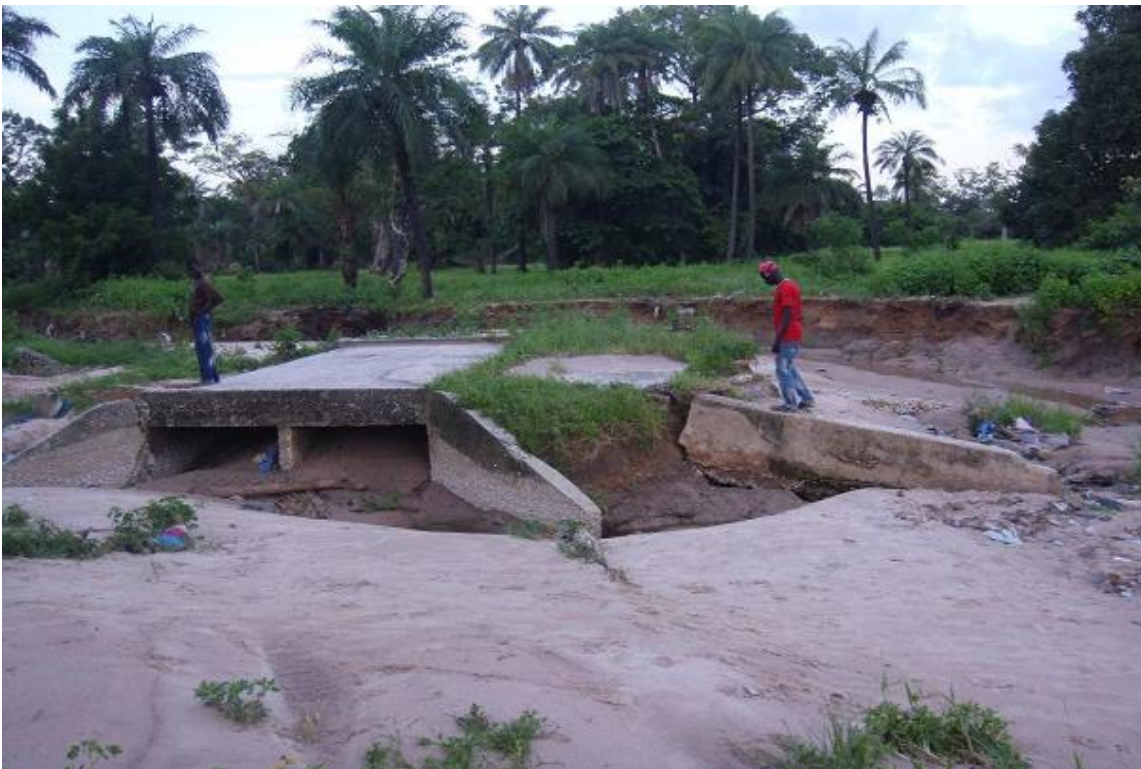
Figure 5: Sanitation system damaged after flooding in Bignona, Senegal (H2O and I&D, 2014).
