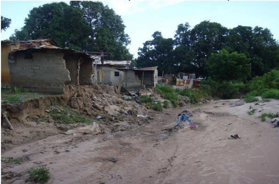
Figure 4: Housing structure damaged by run-off water after heavy rain event (H2O and I&D, 2014).
