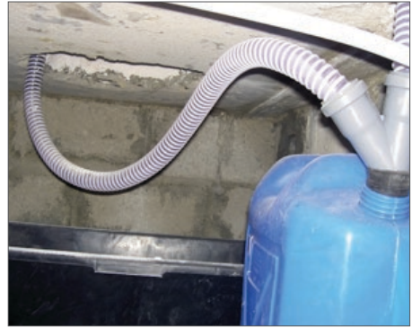
Bad example of urine hose installation, urine stagnating in hose can cause bad smells
