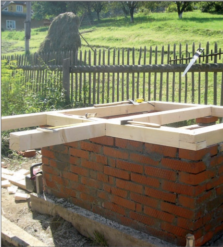
Frame for toilet room floor located on top of the faeces vaults
