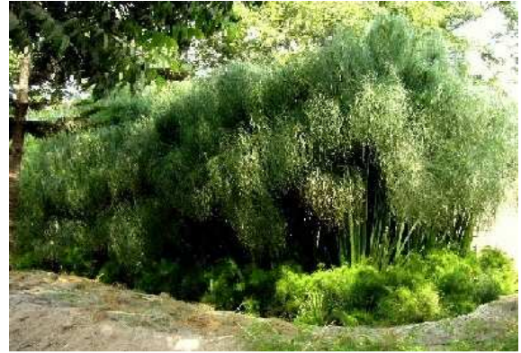
Fig. 8: Vertical flow constructed wetland (reed bed) for treatment of the liquid phase of blackwater (after 6 months of growth)
