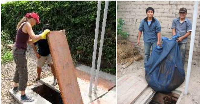
Fig. 6: Double-chamber compost filter ("Rottebehälter") for blackwater pre-treatment (left) and removal of a filter bag (right)
