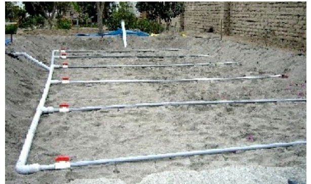
Fig. 18: Distribution system on the second constructed wetland (for blackwater treatment) before planting, showing valves on the left (in red) to avoid clogging (intermittent loading).
