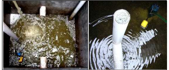
Fig. 4: Outlet of the blackwater compost filter (pre-treatment) (left) and effluent of the constructed wetland (papyrus reed bed) for blackwater treatment (right).
