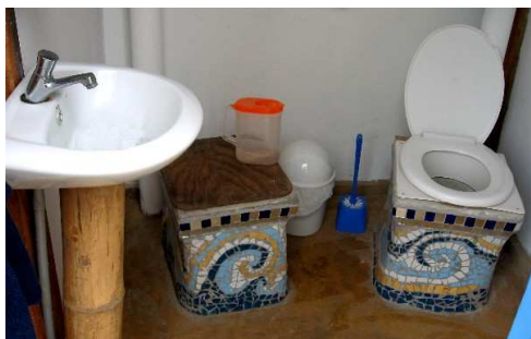
Fig. 10: Inside one UDDT cubicle (Two colourful urine diversion pedestals; only one is in use at a time, for about one year).
