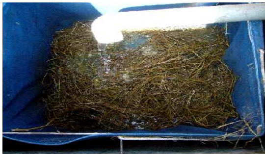
Fig. 17: Increased blackwater flow in the composting chamber (filter bag) due to water leakage in the flush toilets.
