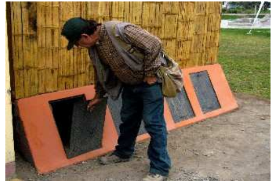
Fig. 11: Two double-vaults for faeces collection at the backside of the UDDT building (4 vaults in total).
