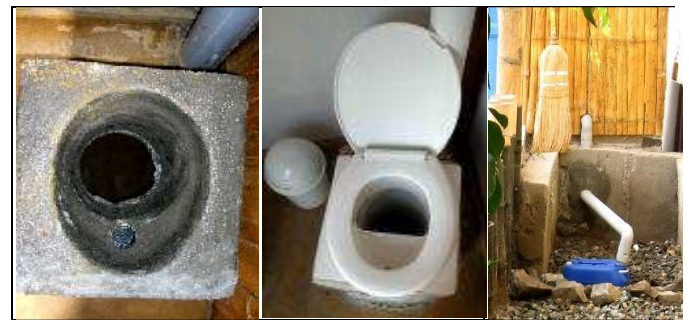
Fig. 12: Toilet seats without (left) and with (middle) plastic insert for urine separation. Pipe from UDD toilet to 25 L urine jerrican (right).
