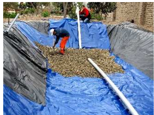
Fig. 3: Drain tube on the base of the constructed wetland for blackwater treatment during covering with gravel. To avoid perforation caused by the gravel, the 0.5 mm PVC liner (in black) needed a special protection. A second liner (in blue) was put inside. 1
