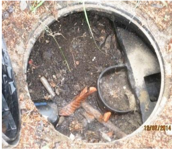
Sludge of septic tank
