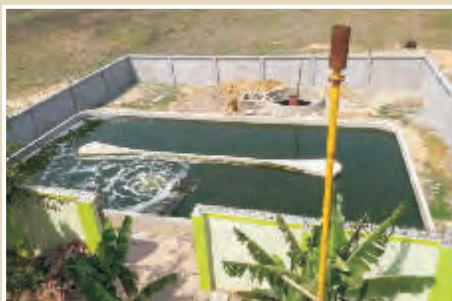
UASB-High Rate Algal Pond combination for black-water treatment SARASWATI Project
