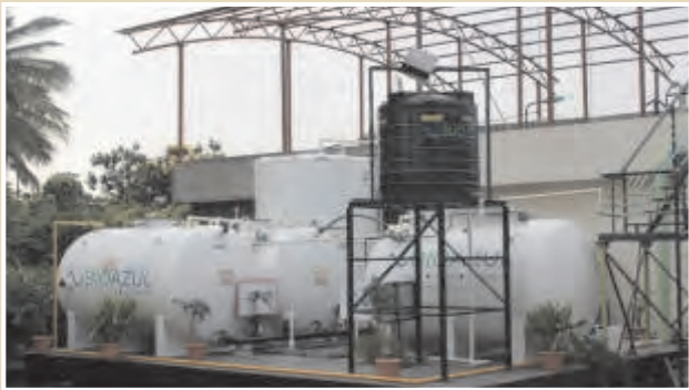
Compact SBR-MBR system at Amanora Park Town- NaWaTech Project
