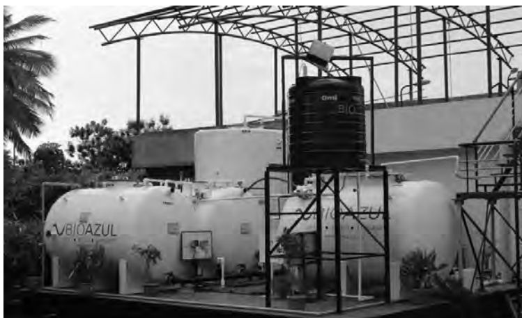
Figure: Compact SBR-MBR system at Amanora Park Town
