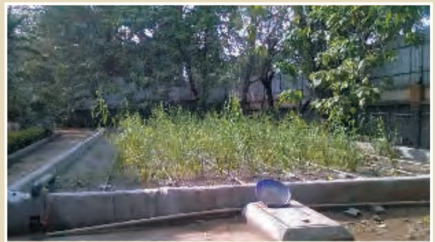
Planted Gravel Filter at COEP-NaWaTech
