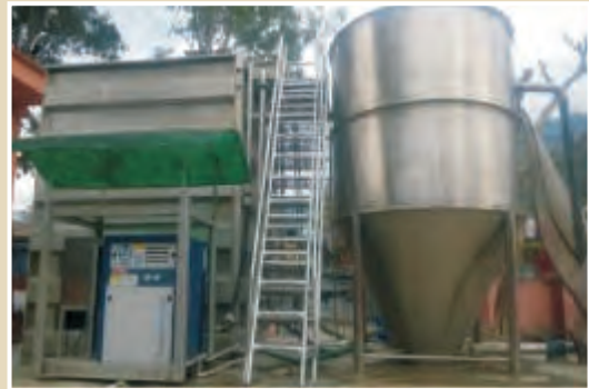
HYSAF Package Plant SARASWATI Project
