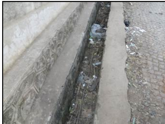
Figure 10: Drainage system (photo credit: Oscar Veses).
