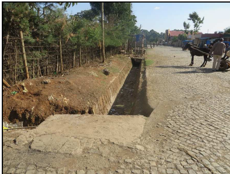
Figure 10: Drainage system (photo credit: Oscar Veses).
