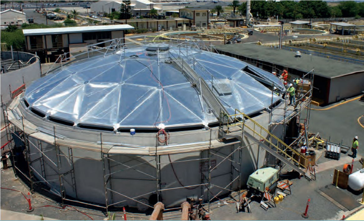
The wastewater treatment plant at the US military's Joint Base Pearl Harbor-Hickam has been retrofitted to capture methane gas for future energy use. Photo: Flickr / US Navy / Denise Emsley
