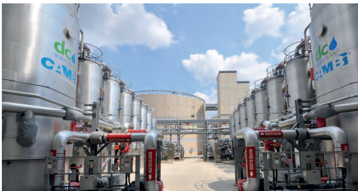
Part of the combined heat and power bioenergy plant at the Blue Plains Advanced Wastewater Treatment Plant, District of Columbia, USA. Photo: DC Water
