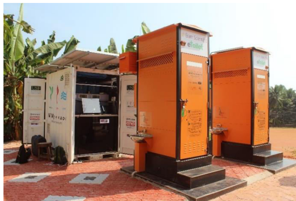
Figure 1: Site picture showing final system as installed at the site. The two orange eToilets can be seen with their associated sinks. The AnMBR housed in a shipping container and PV system can also be seen.
