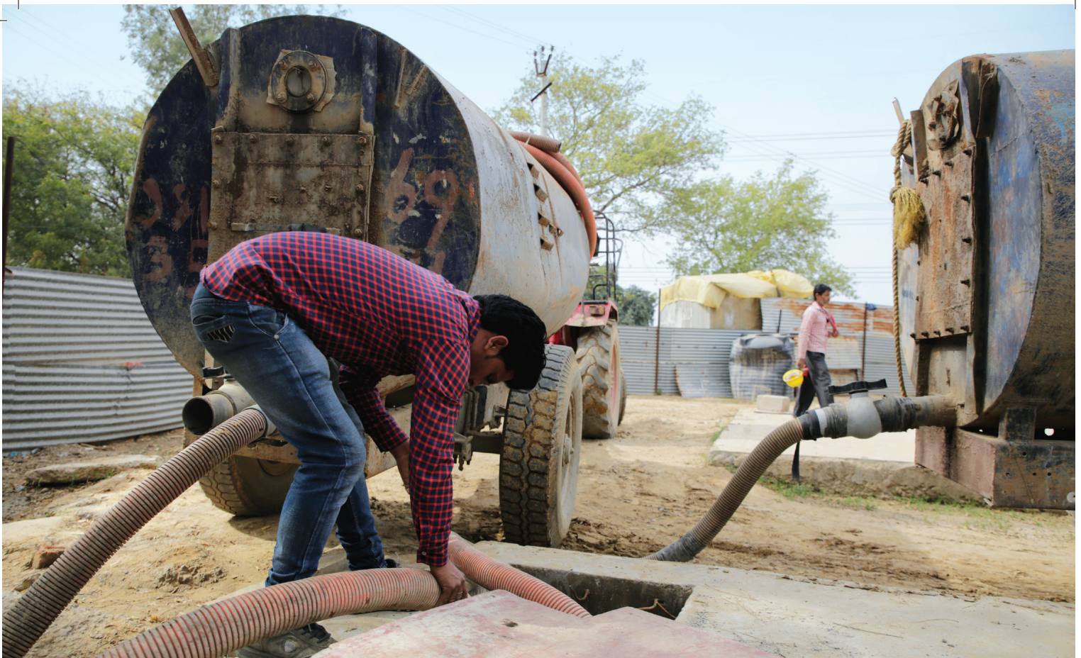
Soak pits at this colony built by a construction company for its workers in Gurgaon have to be emptied every day
