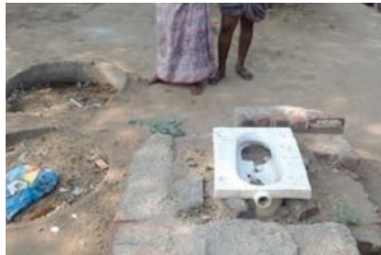
Dysfunctional pit latrine
