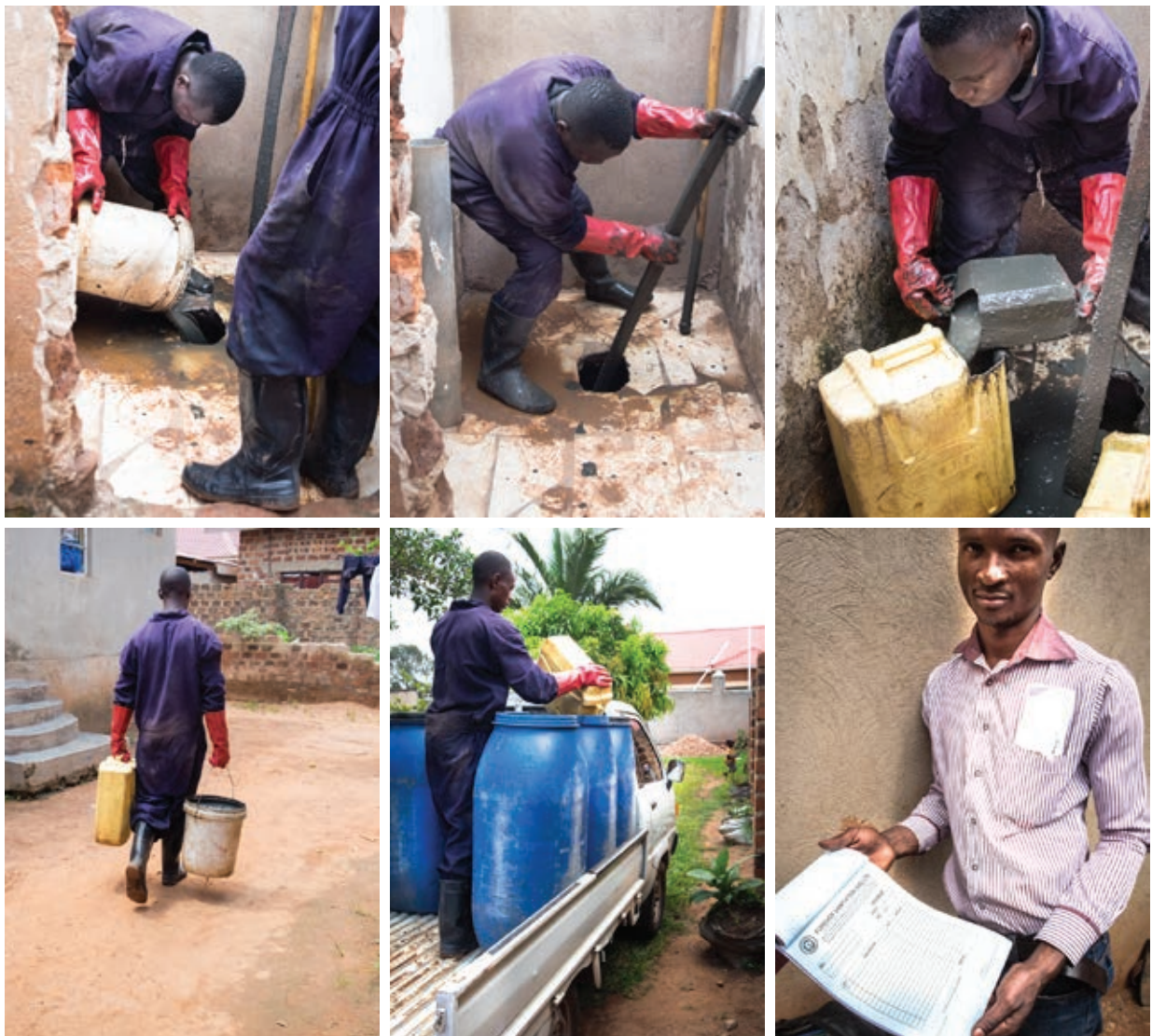
Figure 3: Pit latrine emptying process
