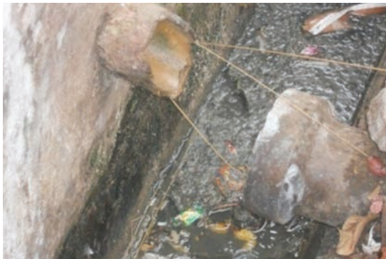
Toilet directly connected to open drain
