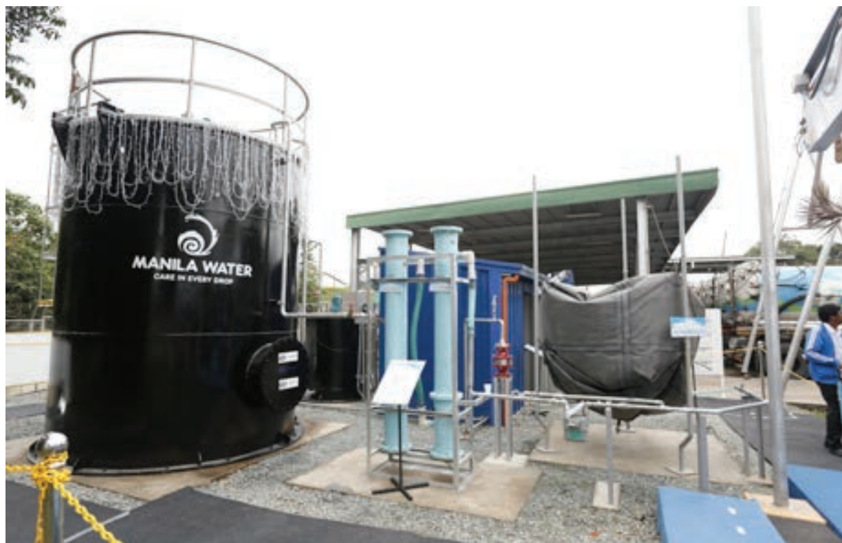
Figure 8: Manila Water’s first Waste to Energy (WTE) septage treatment plant
