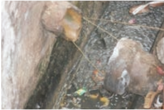
Toilet directly connected to open drain
