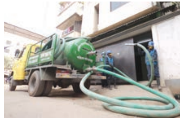
Figure 15: SWEET vacuum tanker in operation in Dhaka
