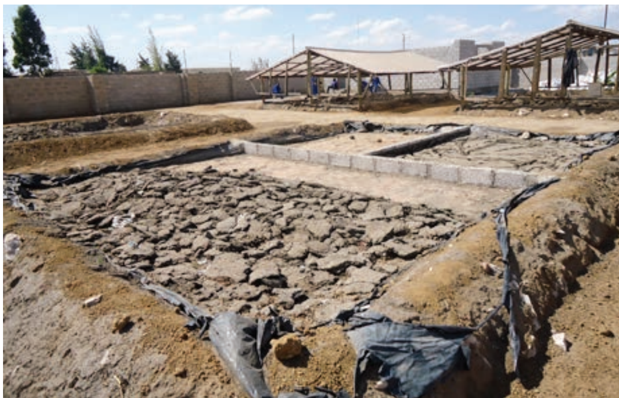
Figure 6: Sludge drying beds
