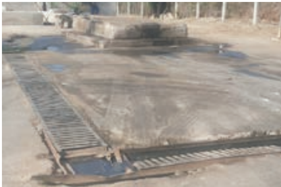
Figure 5: Damaged drain, Rufisque FSTP
