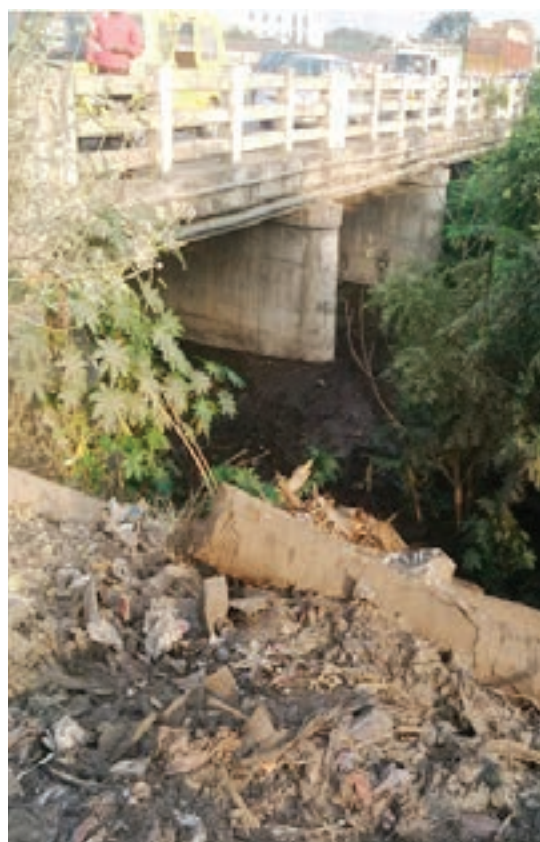
Septage disposal point at Alankar bridge
