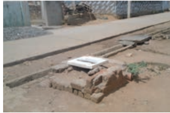
Dysfunctional pit latrine
