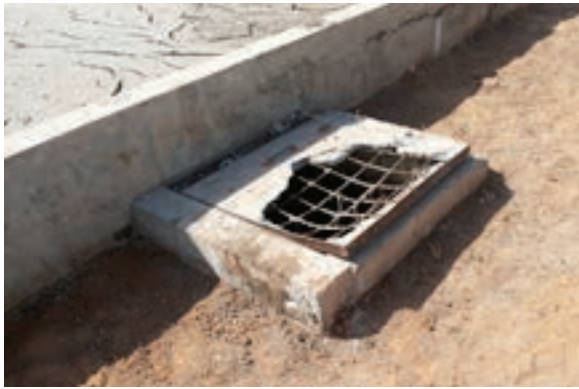
Figure 4: Damaged cover, Cambérène FSTP
