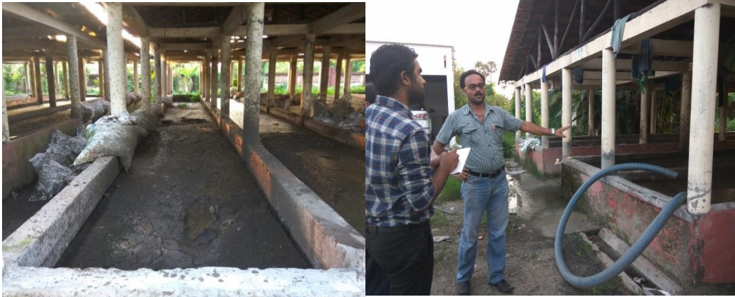
Figure 84: Sludge drying beds (Source: Aishwarya/CSE, 2016)
