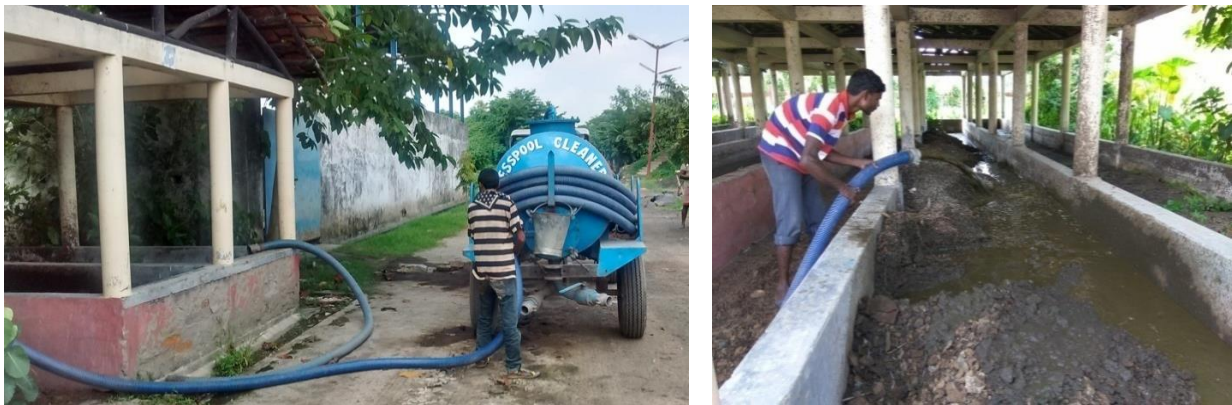
Figure 7: Discharging of septage at FSTP facility (Source: Anil/CSE, 2016)
