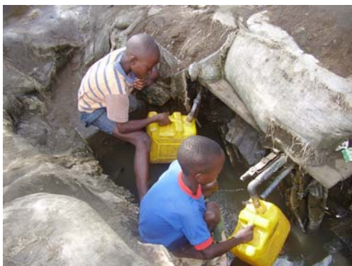
Figure 4-11 Practice resulting from very low pressure in the water distribution mains in John Laing (notice how the a trench is dug to access the main pipe and draw water).
