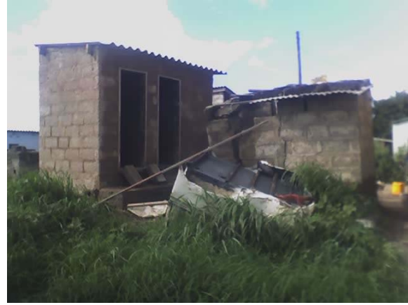
Figure 4-16 New toilet replacing a collapsed one on the right. (in John Laing).
