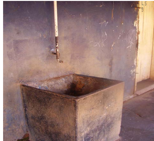
Figure 4-4 Broken hand wash basin outside pupils toilet at the old govt. school
