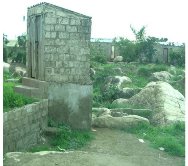
Figure 4-14 Karst geology and raised toilets in John Laing (notice the leak in the side).
