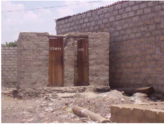
Figure 4-9 A privately built toilet servicing patrons at a bar in Chawama (right near the fee paying toilet/shower shown in Figure 4-10; notice the incompleteness of the structure).
