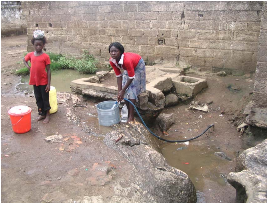
Figure 4-7 Dilapidated stand post with connection on the main pipe to draw water in Chawama (source: (GKW, 2005)).
