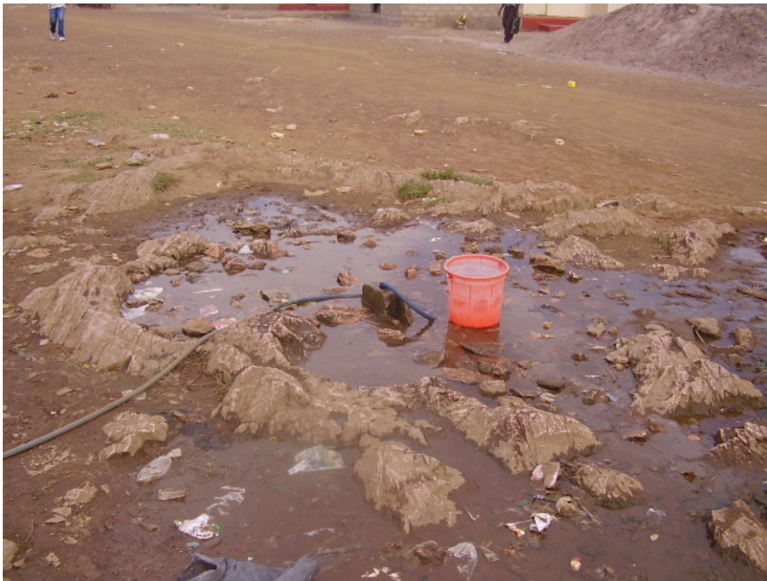
Figure 4-8 Hose pipe connected on saddle clamp on main pipe to draw water in Chawama
