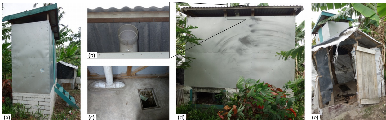
Figure 40: Side view of the Composting Toilet in Salvabay (a). The vent pipe ended below the roof with a 90° bend (b). One vent pipe was used to aerate both vaults and included three 90° bends (b, c). The left vault door was broken (d). A bush-toilet was built next to the Composting Toilet as an temporary replacement (e).
