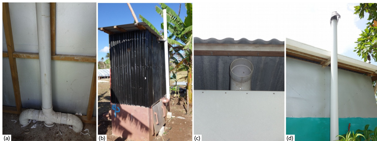
Figure 37: Examples of ventilation systems from Composting Toilets in Vanuatu. All of the inspected toilets had only one pipe for both vaults and included one or more 90° bends, at the junction (a) and (b), or at the top (c). None of them had a rain protection. The ventilation pipe in (c) prevents rain from intruding the vaults, but is not apt for a proper ventilation. (b) and (d) are raised above the roof but the fly screen is poor.
