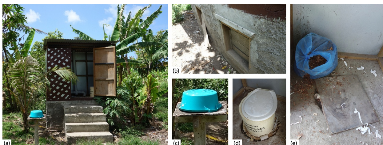
Figure 41: Front view of the Composting Toilet in the Paama community including the ventilation system (a). The door of the active vault was broken (b). A hand washing facility was present next to the toilet (neither water nor soap were available) (c). A prefabricated user interface out of fiber-glass was used (d). Saw dust was present in the toilet, but a vessel was missing. The drop hole cover of the inactive vault was not properly mounted (e).
