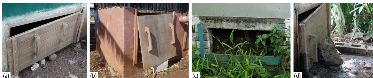
Figure 23: Examples of badly constructed and/or maintained vault doors of 'Composting' Toilets in Vanuatu. The doors are held in position with stones and bricks (a), (b) and (d), or are completely missing (c). Far right (d) shows excessive leaching with pooling due to inadequate usage of cover material in a 'Composting' Toilet.
