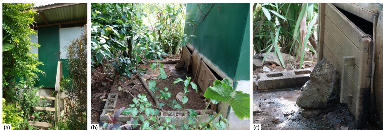
Figure 42: Front of the Composting Toilet in Pepsi (a), the 'infiltration bed' on the backside including the two vault doors (b), and an enlarged view of the vault door from the active vault with liquids pooling in the bed (c).
