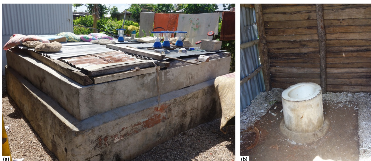
Figure 46: Concrete tank to store rainwater (a) and a Pour-Flush Toilet (b) in Tongamea.
