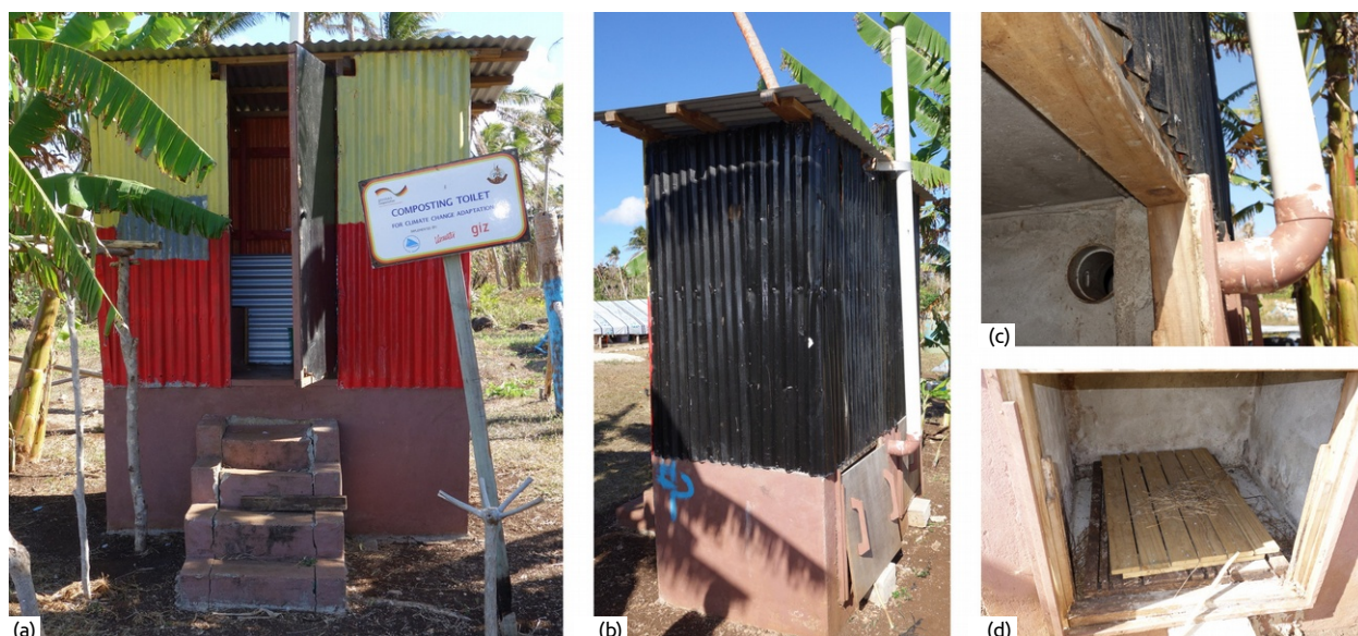
Figure 39: Composting Toilet from the front (a), sideways including vault doors and vent pipe (b), two 90° bends of the vent pipe (c) and the false floor in the unused vault (d).
